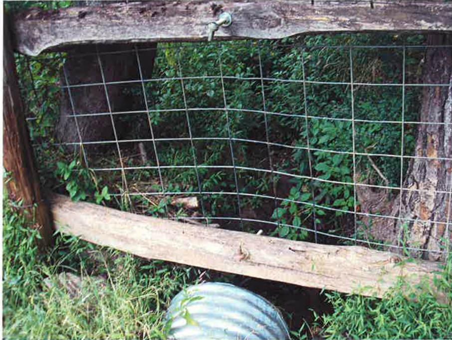
Cattle Crossing Photo - 1 UT1 as it enters culvert of newly constructed cattle crossing. (EMH&T, 9/16/11)
