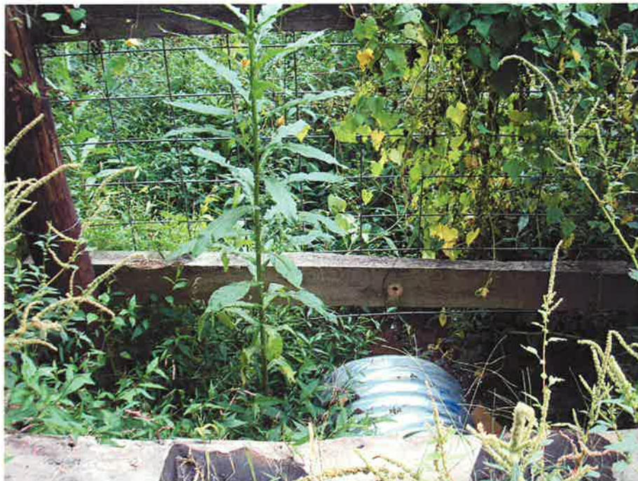
Cattle Crossing Photo - 2 UT1 as it exits culvert of newly constructed cattle crossing. (EMH&T, 9/16/11)
