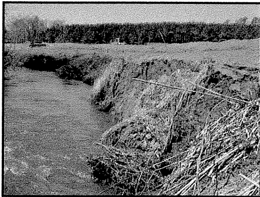
Photo 11 – Streambank erosion along AR1
