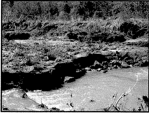
Photo 1 – Eroding bank along SR1
