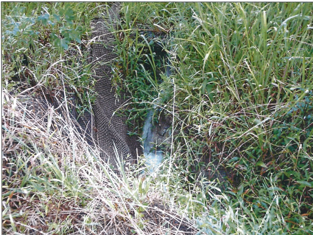
Close-up of erosion behind CV
