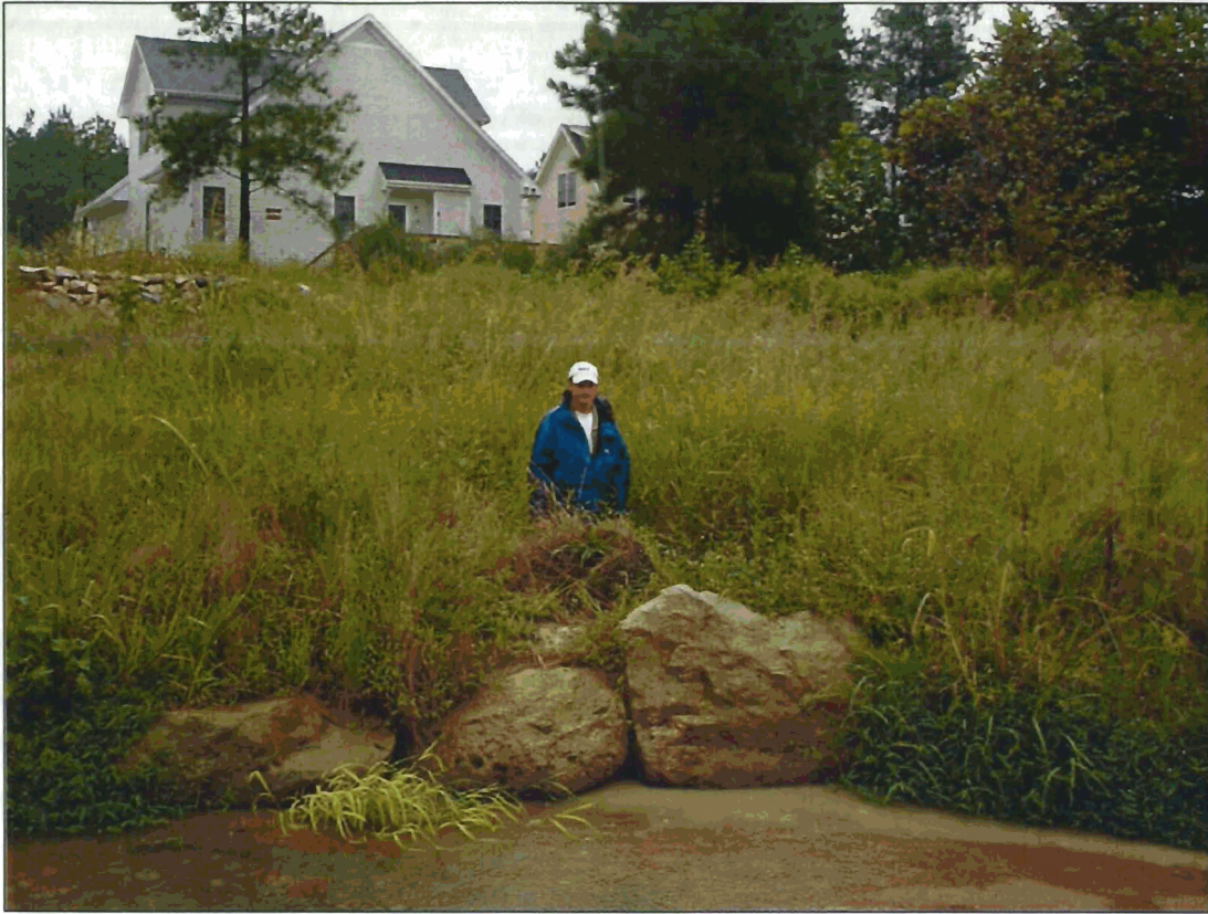
Erosion behind CV on AR3 STA 37+15 due to storm water outlet
