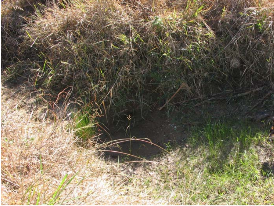
VPA3 Smith Creek Station 38+60. Gully in floodplain from overland flow.
