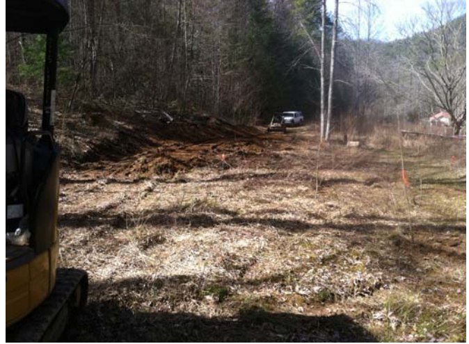
VPA2 – New path being graded to move access road outside of the easement and eliminate easement encroachment. View looking downslope from above easement alignment.
