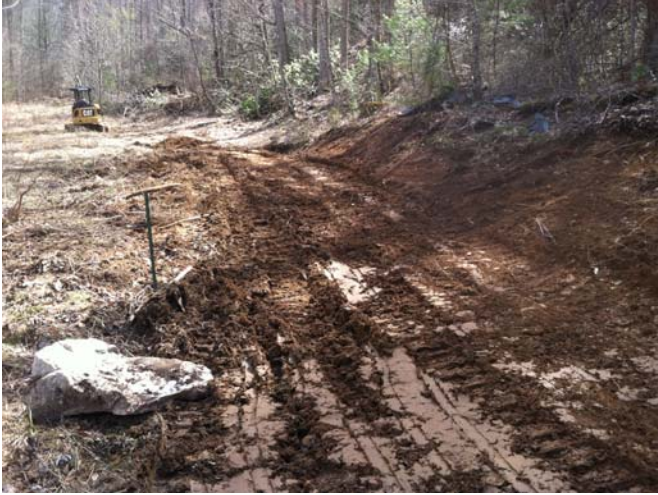
VPA1 – New path being graded to move access road outside of the easement and eliminate easement encroachment. View looking upslope from near the stream crossing.
