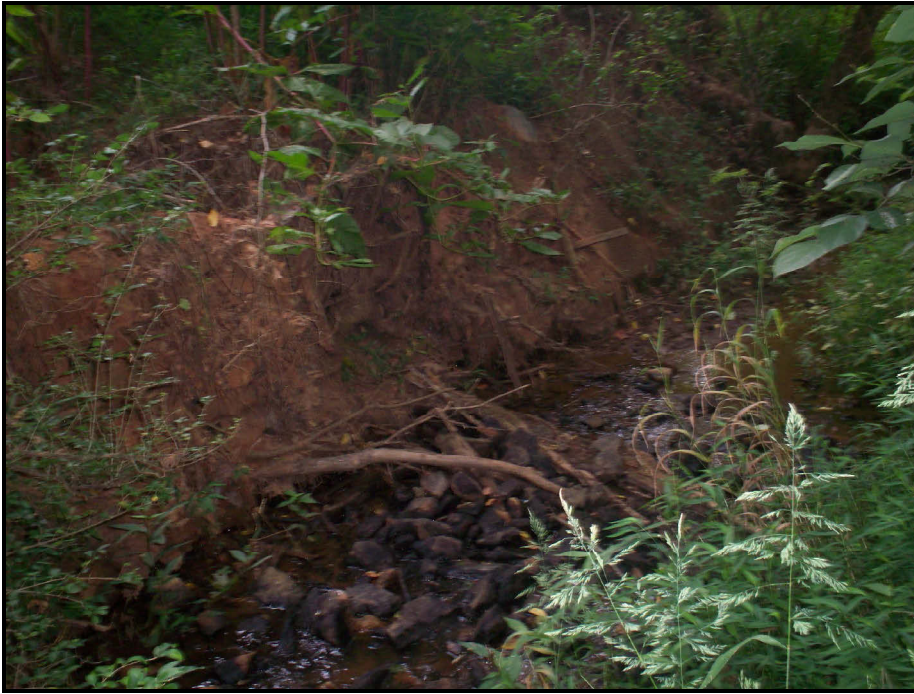
SPA 1. Erosion along left bank in UT-2A North at STA 10+50
