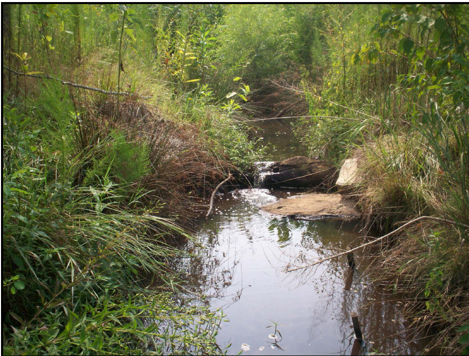
SPA 12. Water backing up below Log weir and over constructed riffle in M2 South at STA 31+00.
