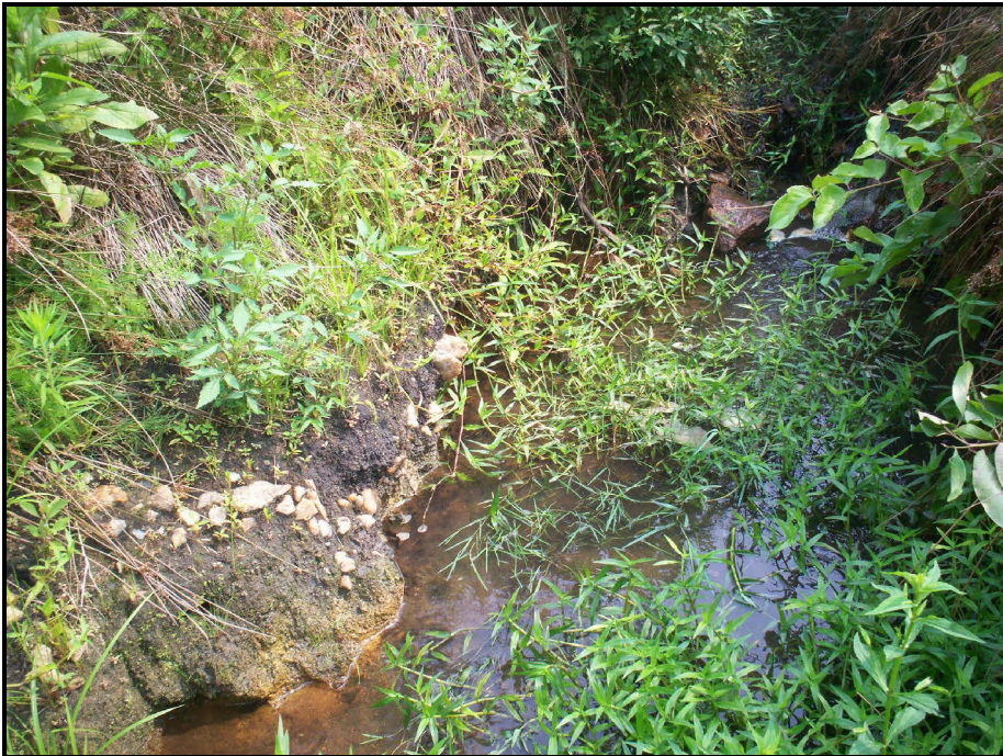
SPA 14. Bank incision downstream of head cut in M2 South at STA 37+50.
