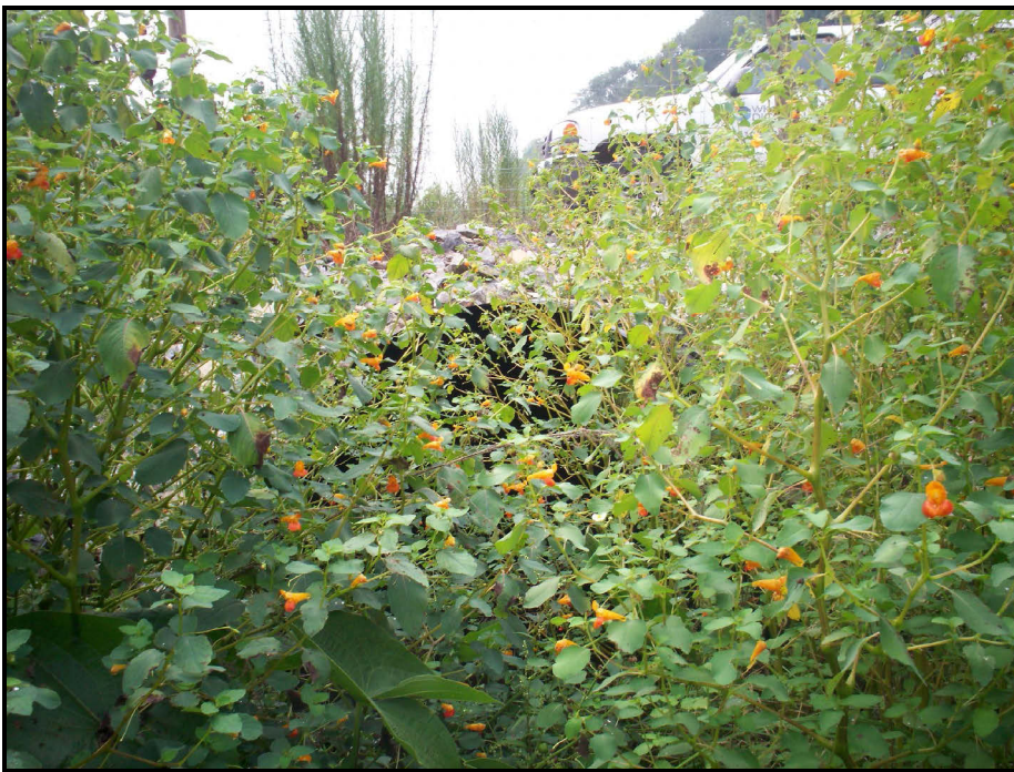
SPA 2. Aggradation mid-channel below culvert and vegetation growing in the channel in UT 2A North at STA 15+50 and throughout upstream section of UT 2A
