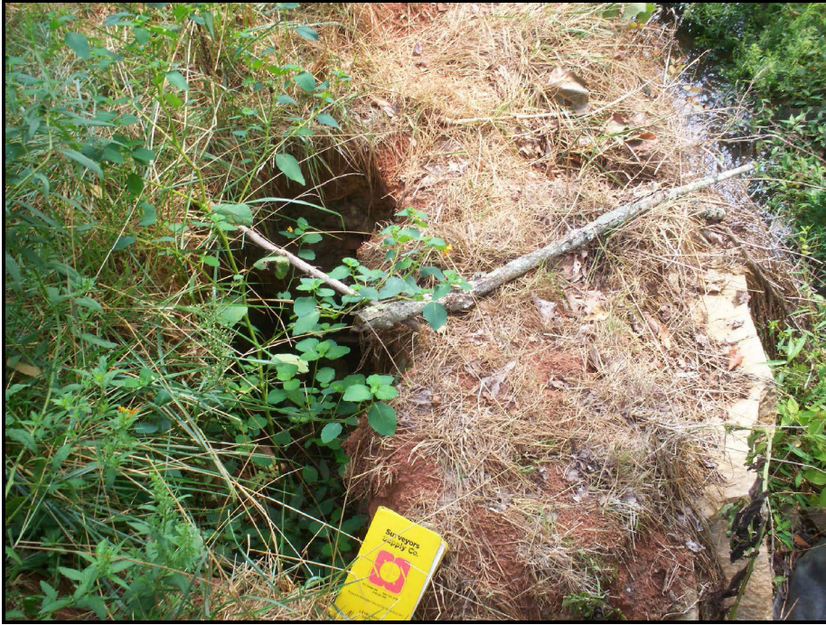
SPA 15. Erosion behind boulder at step pool in M2 South at STA 38+00
