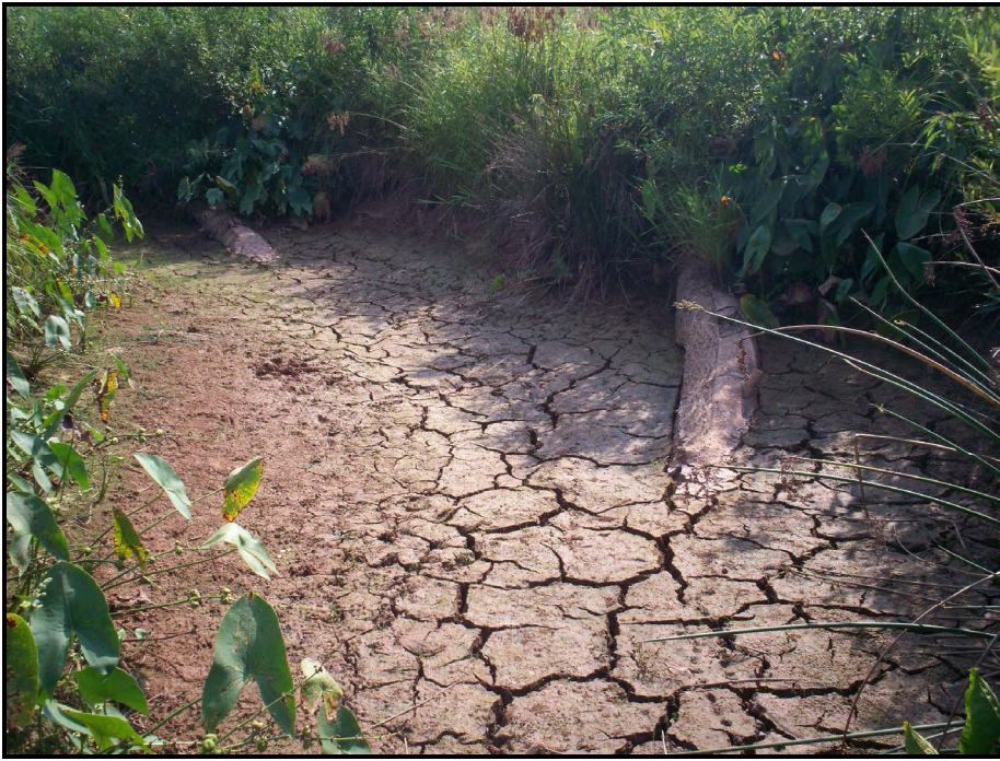
SPA 5. Log vanes buried by sediment in UT2A North at STA 33+00.
