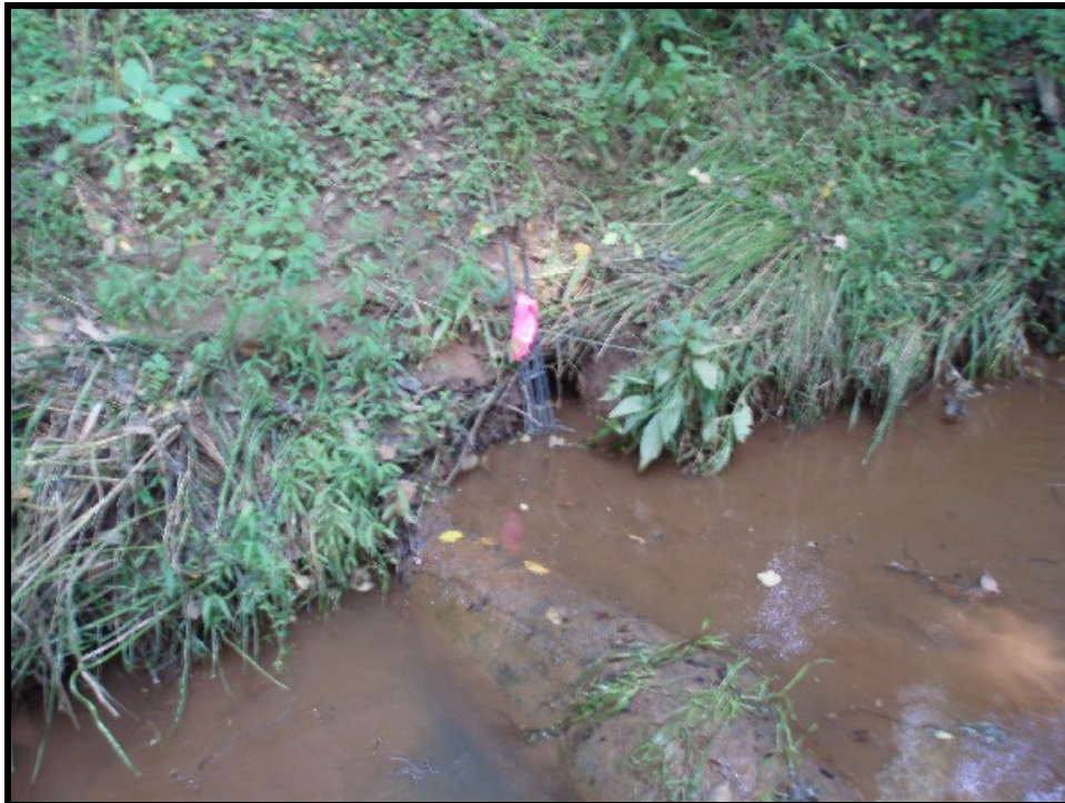
UT1B station 37+60. End cut on right bank at grade control structure.
