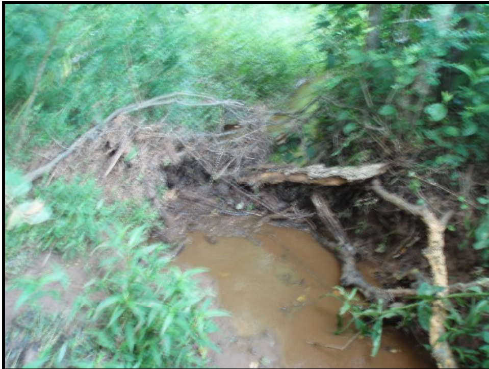
UT1A station 13+00. Small debris jam.
