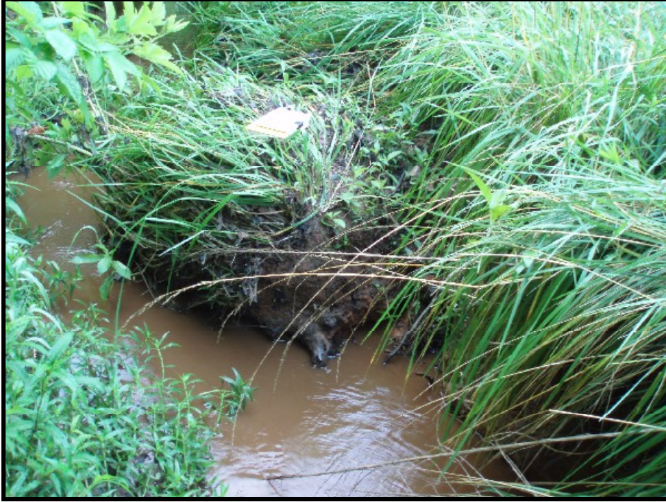
UT1A station 14+80. Slump on right bank.
