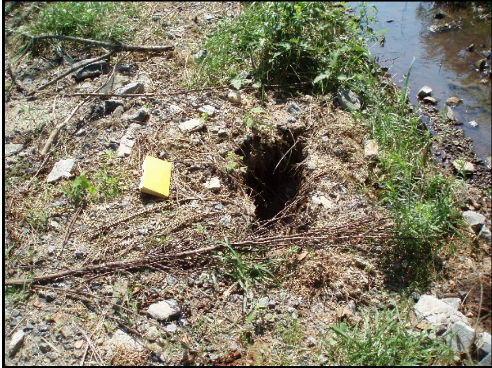
M2 station 38+20. Erosion/settling on right bank.
