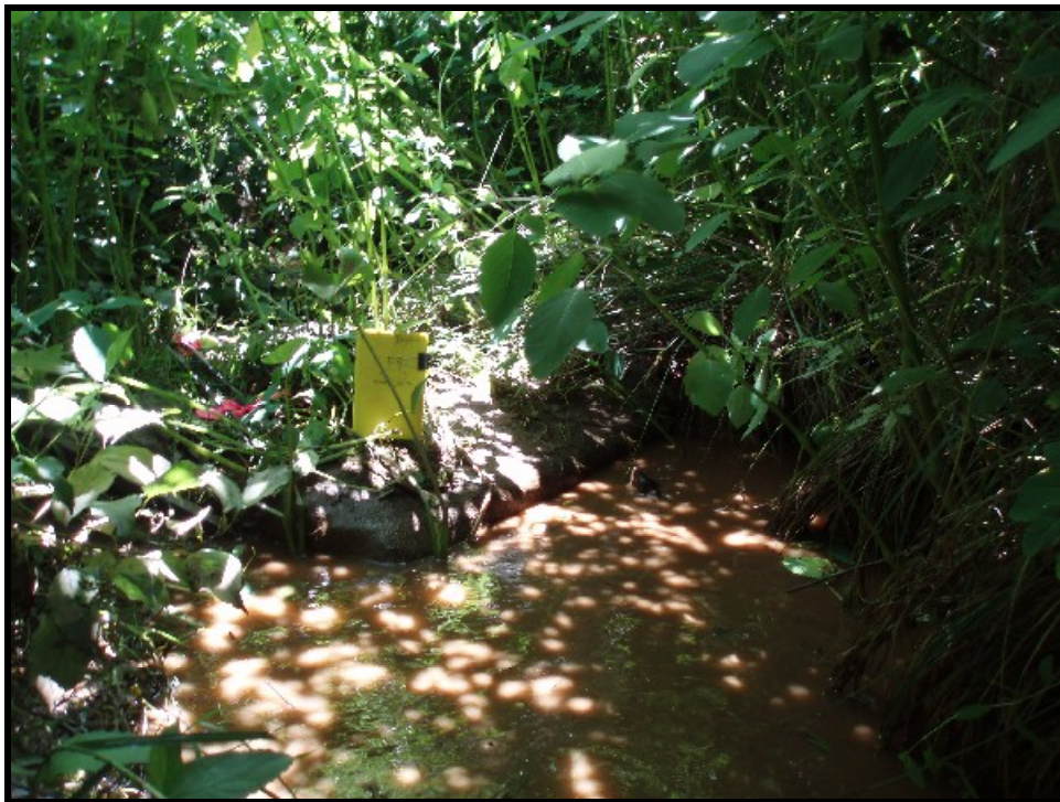
UT2A station 18+90. Rock cross vane header perched.
