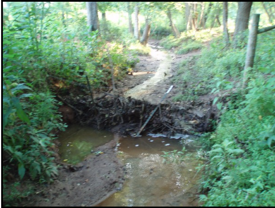
UT1A station 10+00. Wrack in fence.
