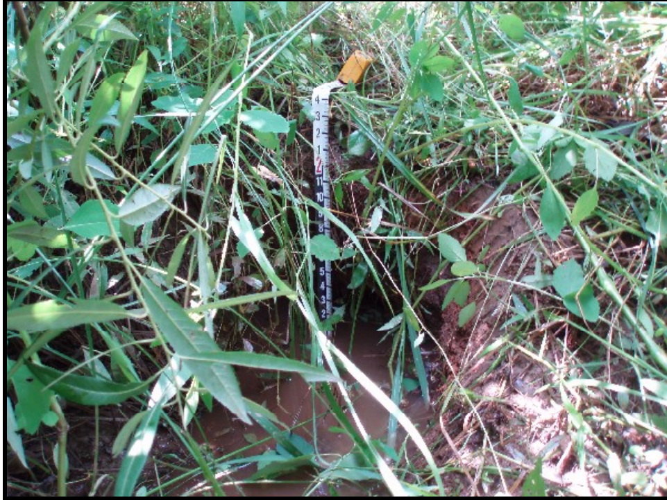
UT2A station 17+60. Left bank erosion.
