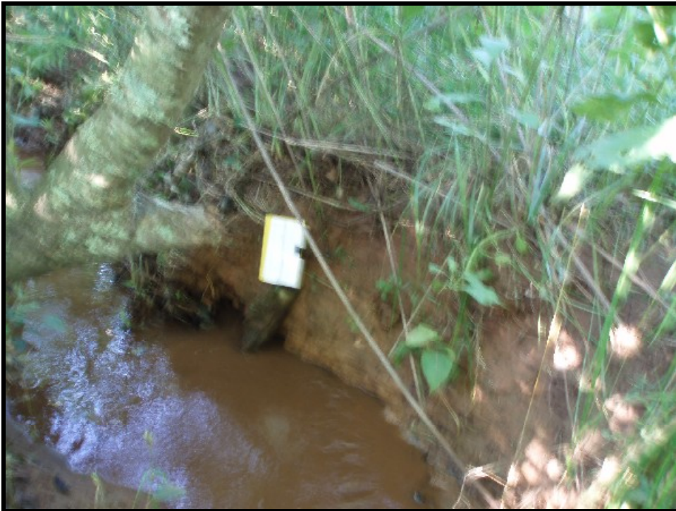
UT1A station 19+00. Typical bank erosion.
