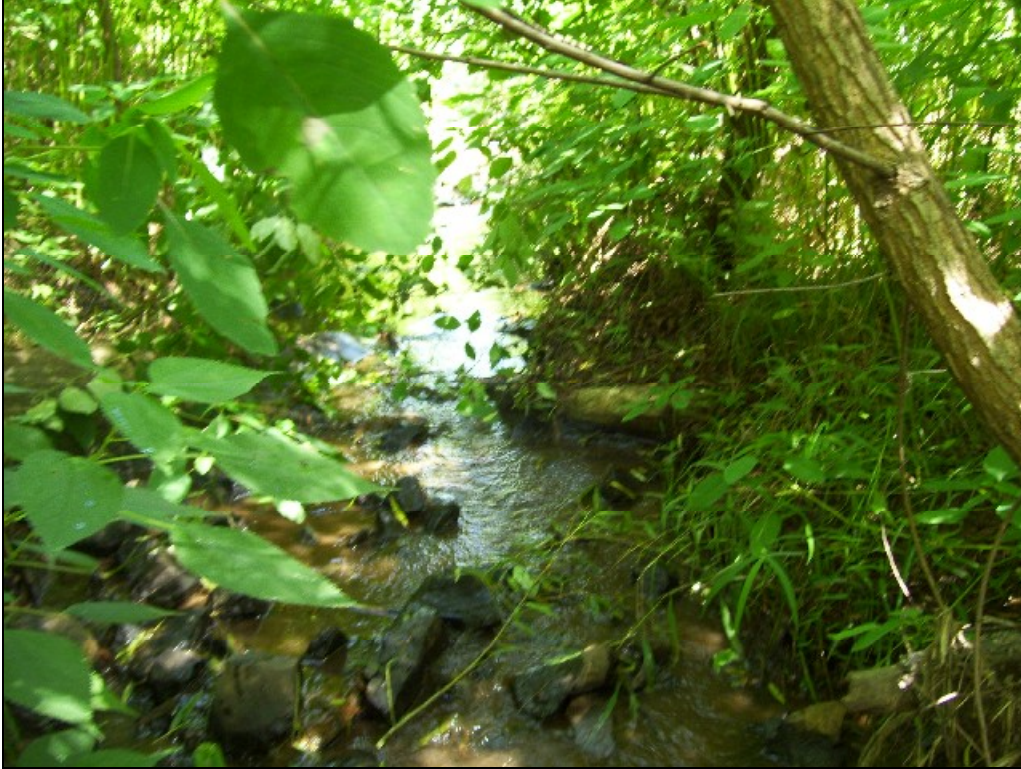
M2 STA 30+90 Minor piping beneath constructed riffle header rock
