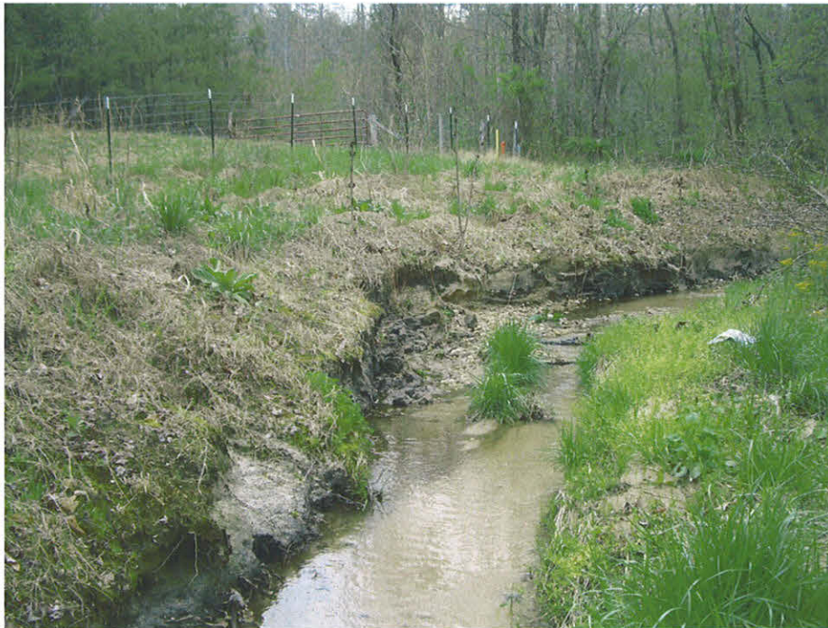
SPA 6 Bank scour along Tributary C at station 15+70. (EMH&T, Inc. 4/14/07)
