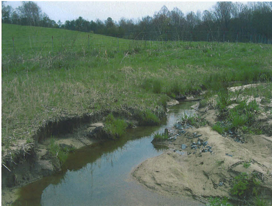
SPA 2 Bank failure along Tributary B at station 12+10. (EMH&T, Inc. 4/14/07)
