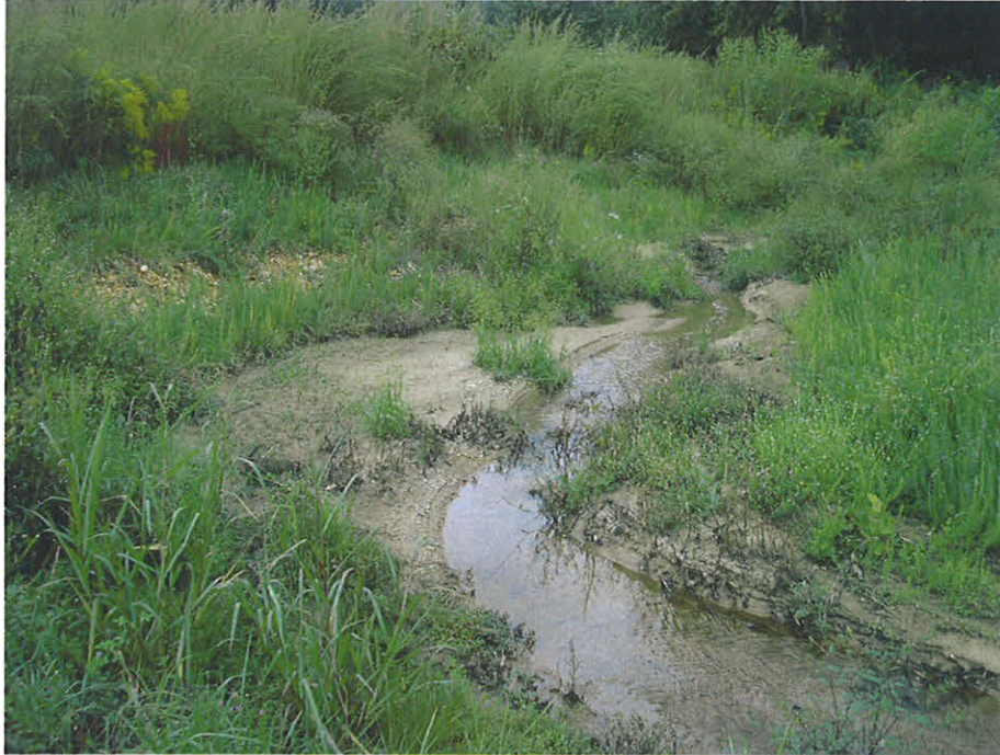
SPA 1 Aggradation in Tributary A2 at station 3+00. (EMH&T, Inc. 9/19/06)
