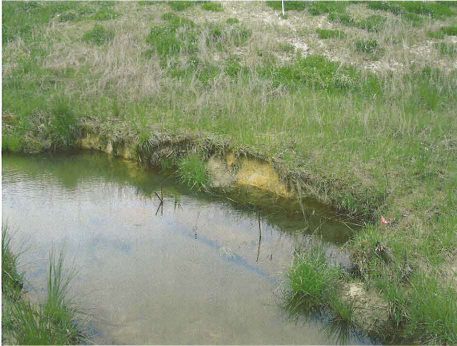
SPA 5 Bank scour along Tributary A (middle) at station 83+30. (EMH&T, Inc. 4/14/07)
