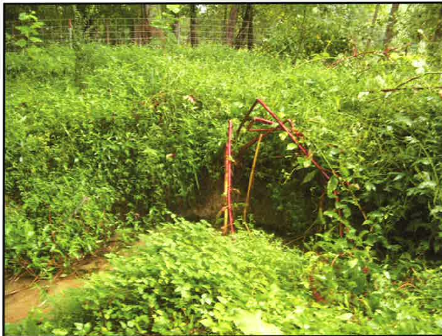
SPA 4 Close-up of bank scour along the right bank of Tributary C near station 4+11. (EMH&T, Inc. 9/16/09)
