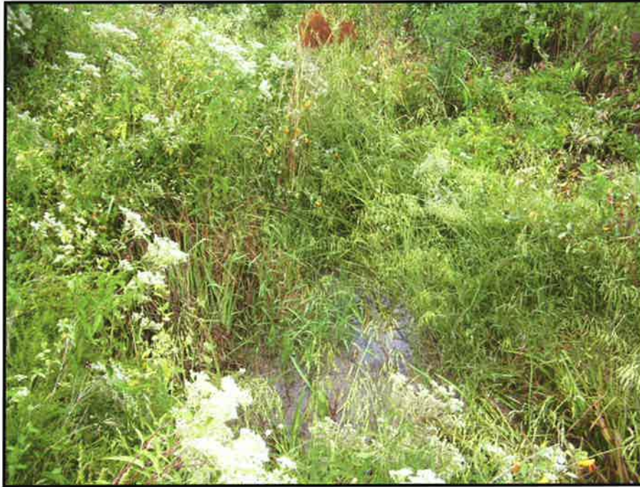
SPA 3 Slumping of the left bank on Tributary A (middle) near station 84+75. (EMH&T, Inc. 9/16/09)
