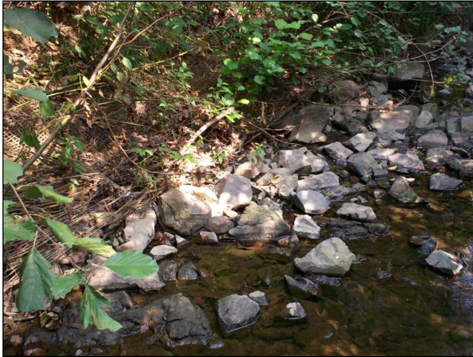
Problem Area # 1. Coir matting failure. Station 11+50 Left bank.
