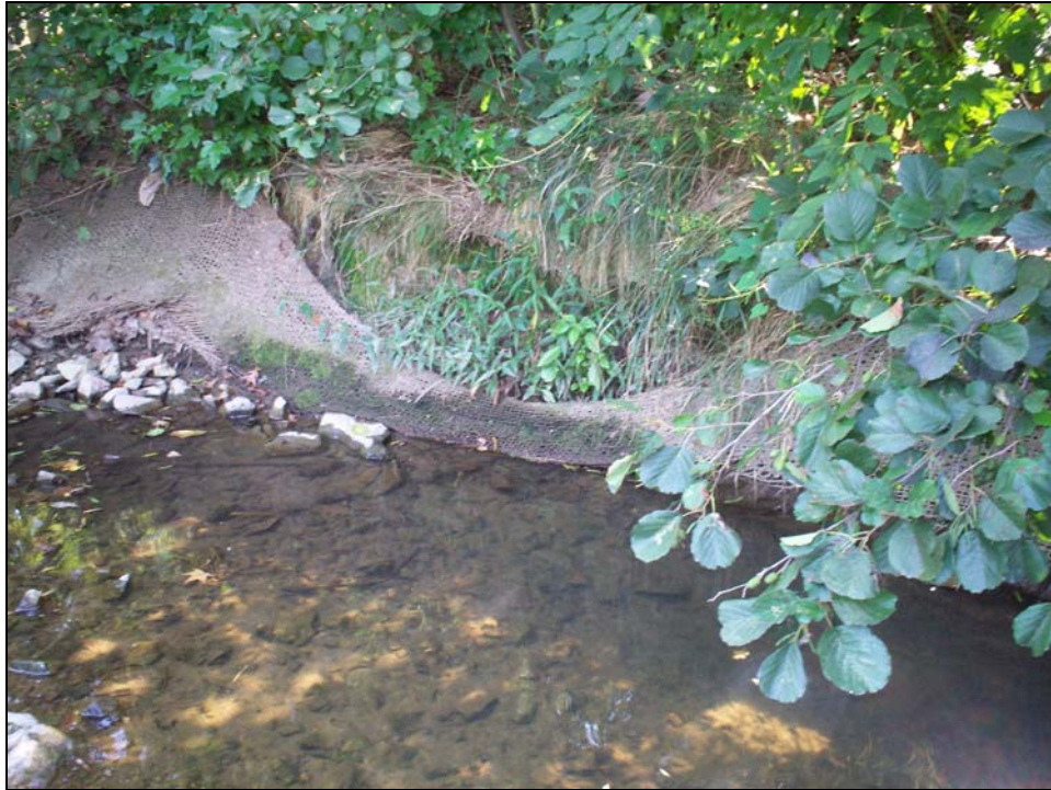
Problem Area #9. Coir matting failure. Station 17+50 Right bank.
