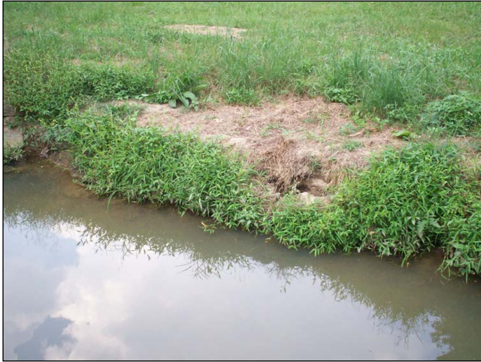
Problem Area # 15. Erosion and mass wasting along left bank due to lack of adequate buffer. Station 18+75 Left bank.
