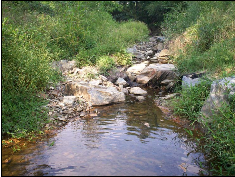
Problem Area #7. Cross vane header moved downstream. Station 17+10 Upstream.
