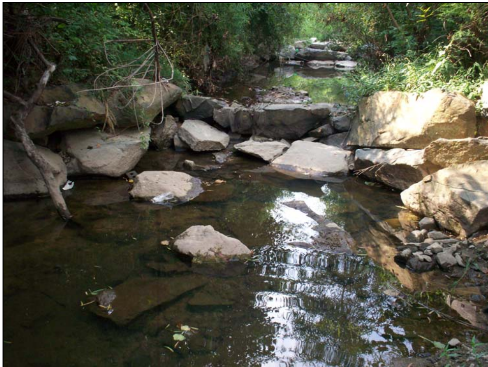
Problem Area # 4. Header on rock vane too high. Station 15+15 Upstream.
