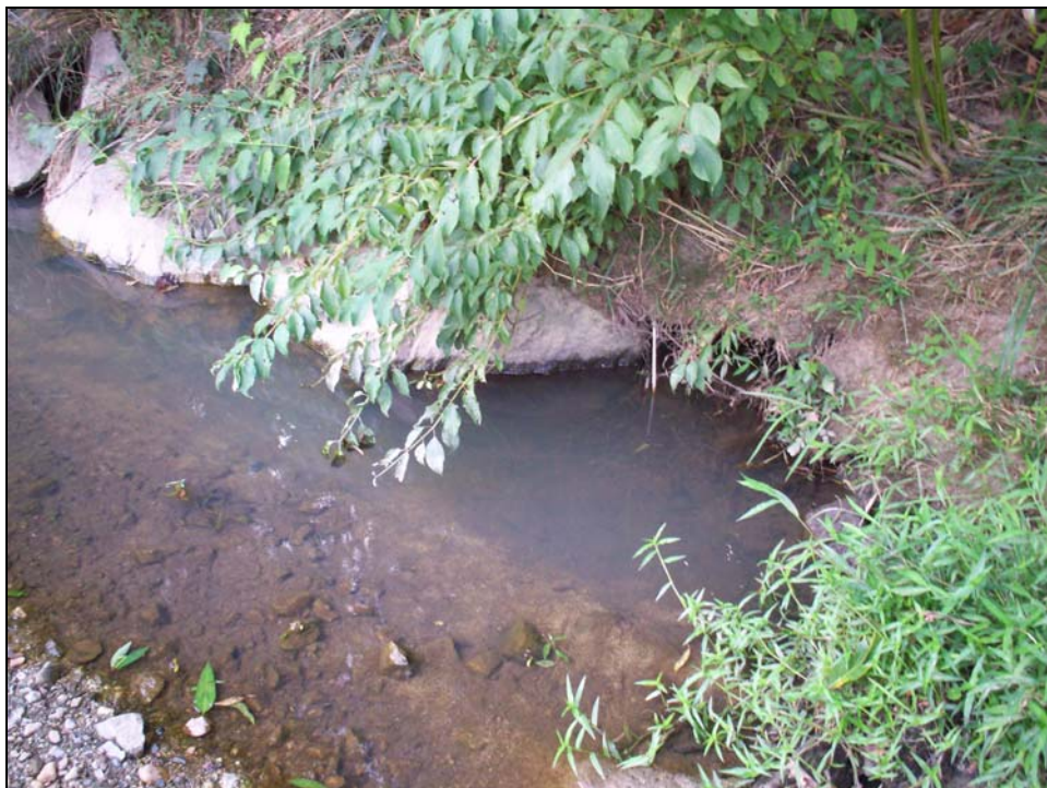
Problem Area # 14. Minor erosion behind gabion wall. Station 19+20 Right bank.
