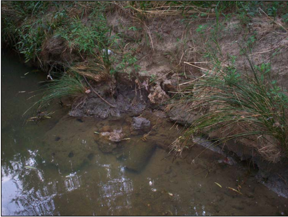
Problem Area # 17. Unstable banks due to erosion. Station 20+30 Right bank.
