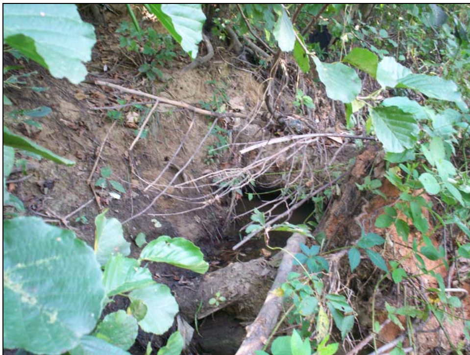
Problem Area #8. Erosion behind root wad. Station 17+15 Right bank.
