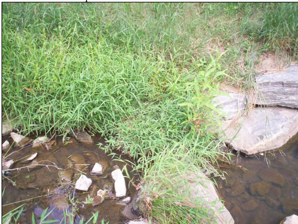
Problem Area # 16. Erosion behind rock vane arm. Station 20+20 Left bank.
