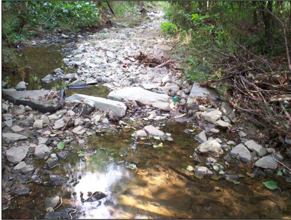
Problem Area # 5. Header on rock vane too high. Station 15+75 Downstream.
