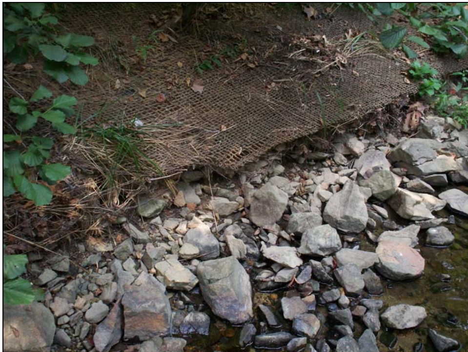
Problem Area # 2. Coir matting failure. Station 13+20 Left bank.
