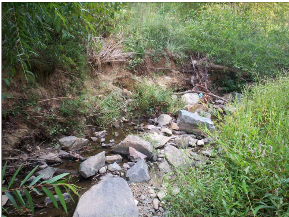
Problem Area #6. Left bank erosion. Station 16+80 Left bank.
