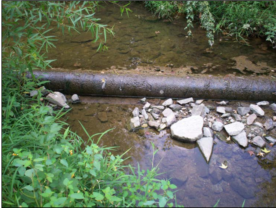
Problem Area # 3. Sewer line exposed. Station 14+40 Upstream.
