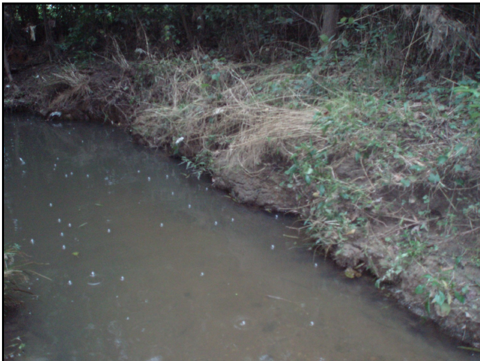
PA #10 – Right bank erosion; lack of rooted vegetation. Sta. 22+80 to 23+00
