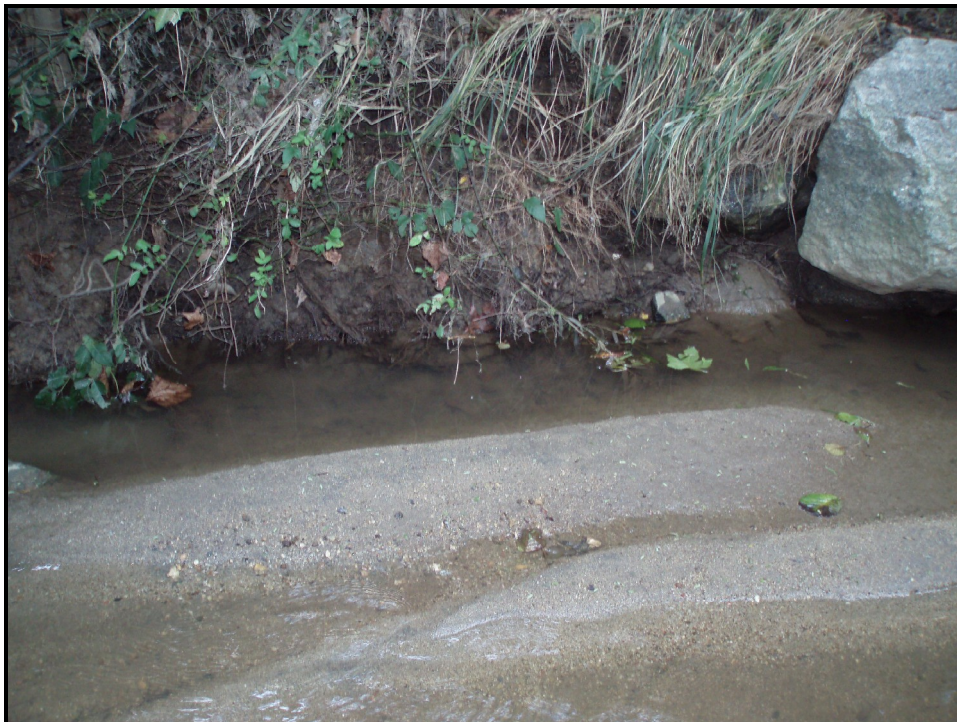
PA #6 – Right bank erosion; lack of rooted vegetation. Sta. 18+40
