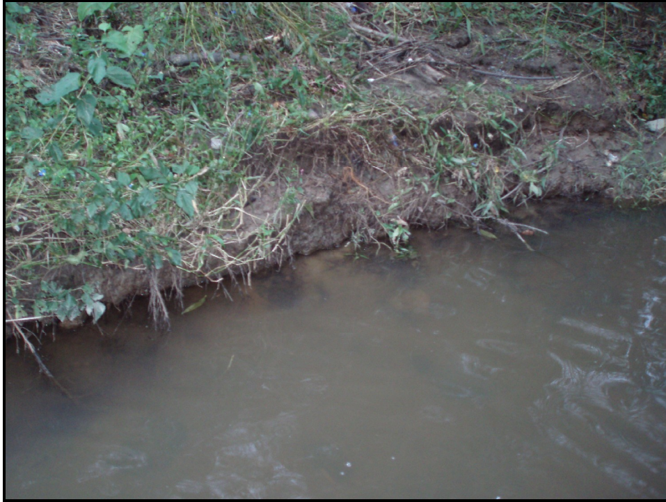
PA #9 – Minor left bank erosion; lack of rooted vegetation. Sta. 21+80
