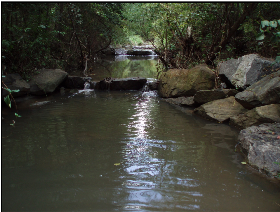
PA# 2 – Cross vane not functioning as intended. Sta. 14+40
