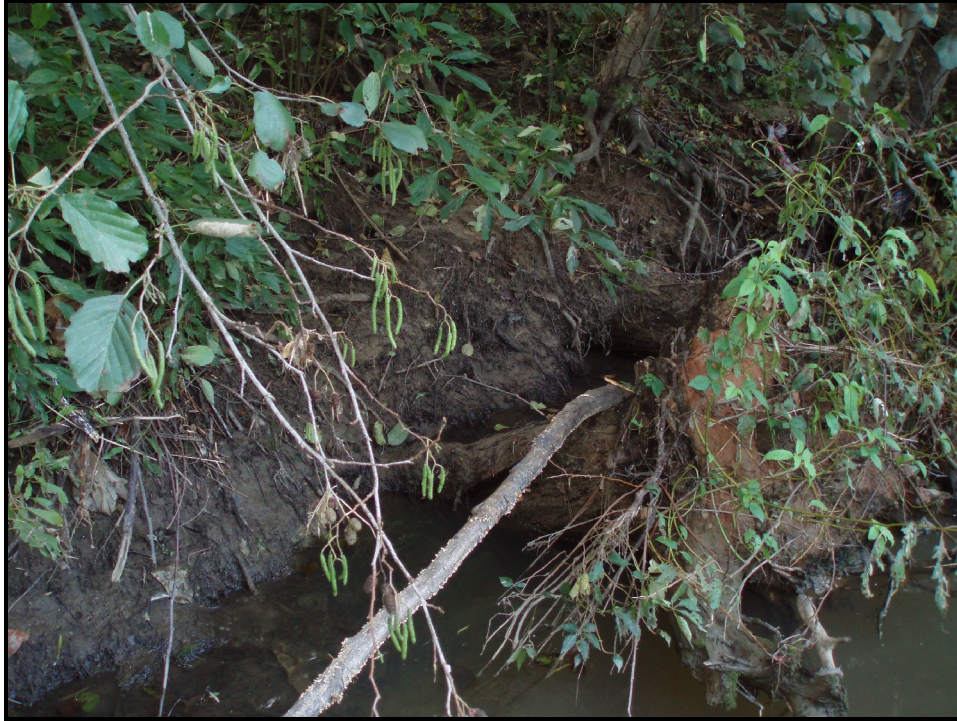
PA #5 – Right bank washed out behind root wad; improper installation. Sta. 17+40
