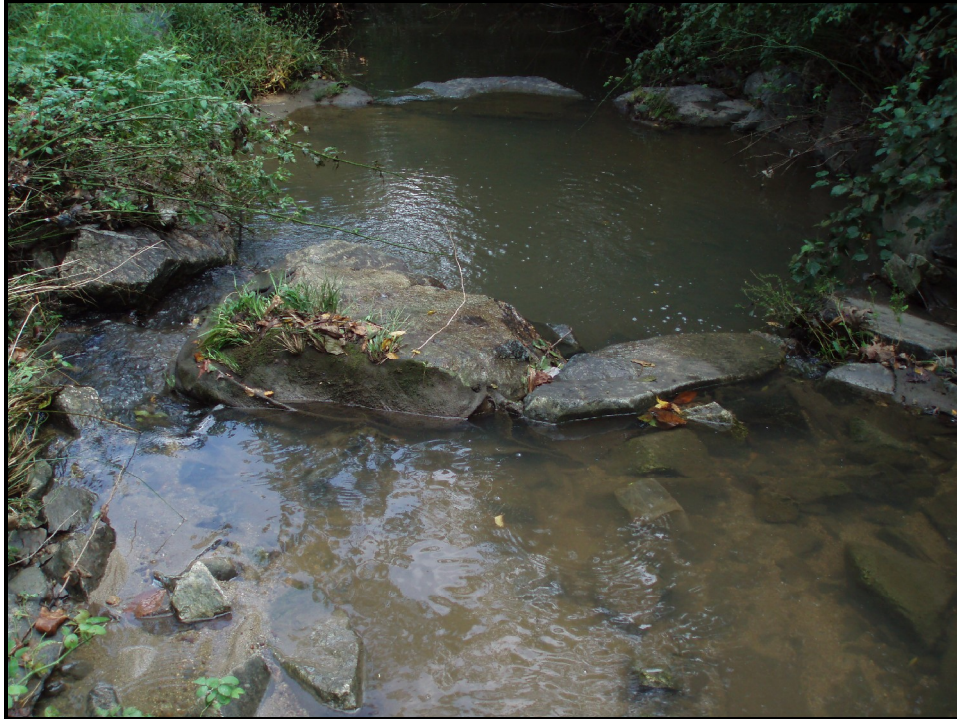
PA #1 – Header on cross vane set too high, water flowing around due to improper installation. Sta. 14+15
