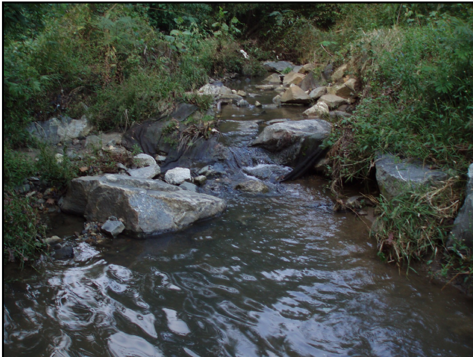
PA #4 – Header rock moved downstream from cross vane; improper installation. Sta. 16+90
