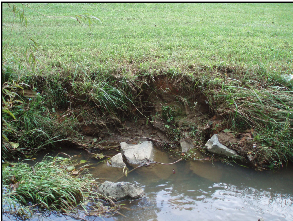
PA #8 – Left bank erosion; lack of rooted vegetation. Sta. 19+00
