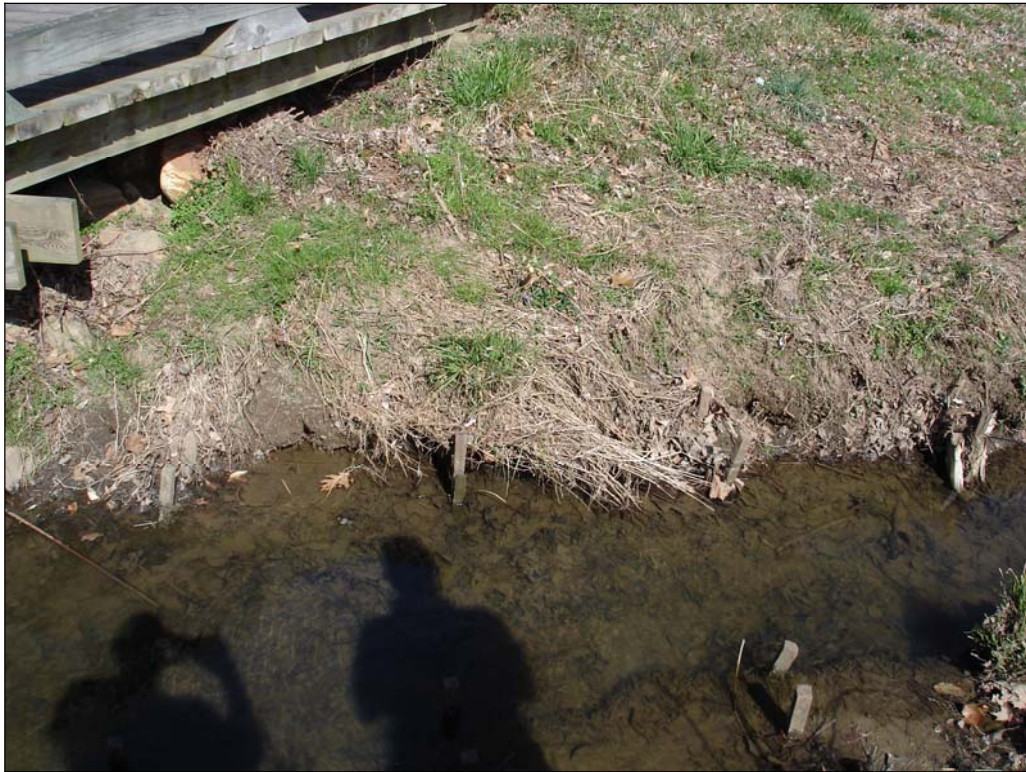
Starmount Forest 2006, Thread D, minor bank erosion at STA 4+80.
