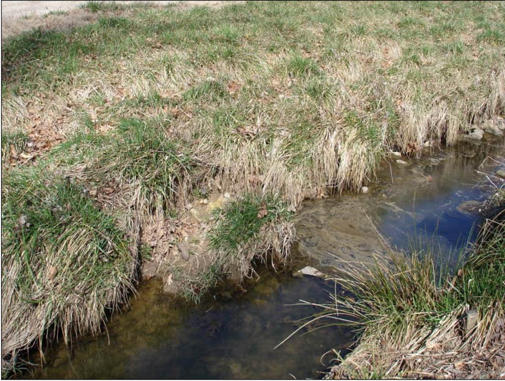
Starmount Forest 2006, Thread D, minor bank erosion at STA 7+10.
