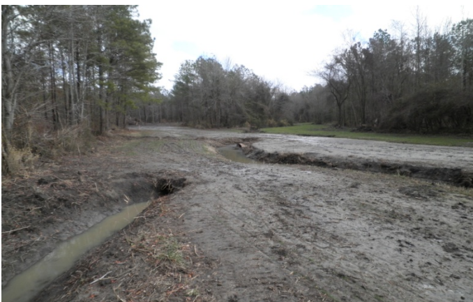
View looking downstream at the existing culverts at the proposed end of UT2
