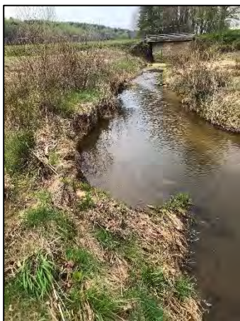
Moores Fork Reach 3, Sta. 49+00 RB Erosion – MY3 (4/13/2022)
