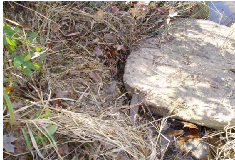
SP2. Piping under cross-vane
