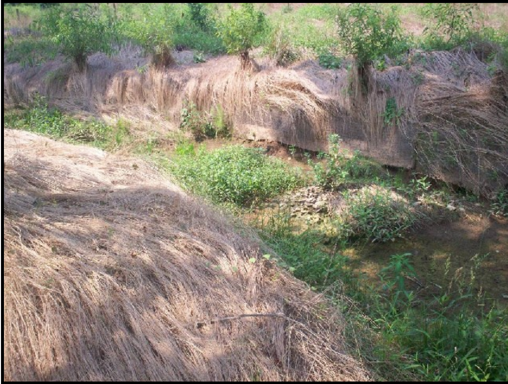
Photo 29. SPA 4. Minor erosion beneath matting; outside of a bend at STA 19+65.
