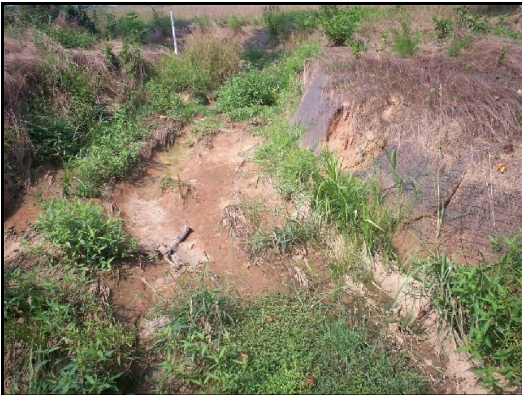
Photo 26. SPA 1. Erosion control matting deteriorating and tearing from slope at STA 1+50.
