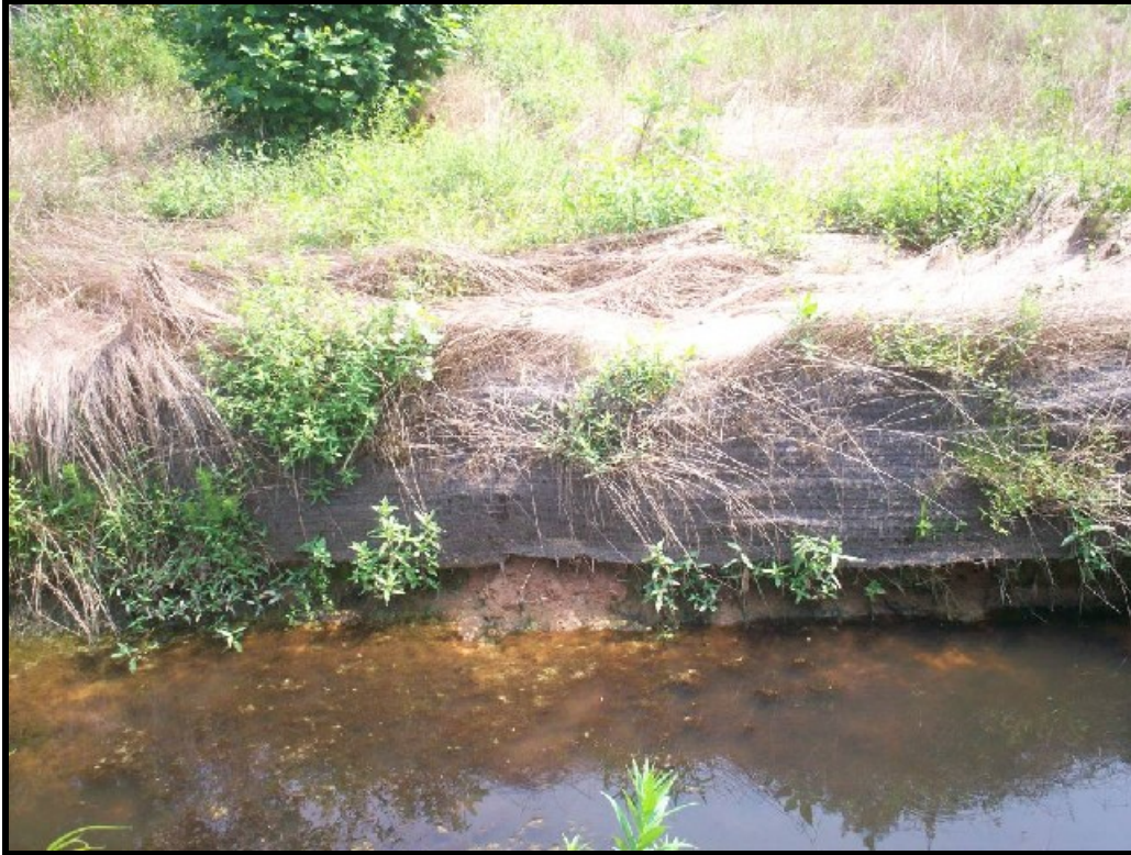
Photo 27. SPA 2. Minor erosion occurring beneath the erosion control matting at STA 12+00.
