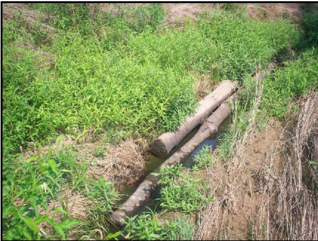
Photo 28. SPA 3. Log toe protection footer log washing out (facing downstream) at STA 16+25.
