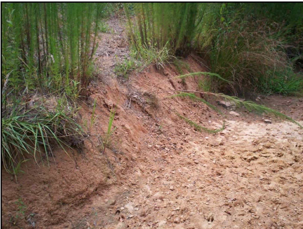
Photo 24. SPA 2. Right bank erosion caused by deer and sparse vegetation at STA 46+90.
