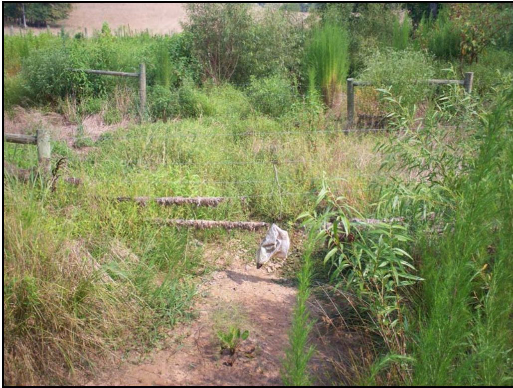
Photo 3. Ford crossing-looking downstream; debris collected on fence from high flows at STA 7+75.
