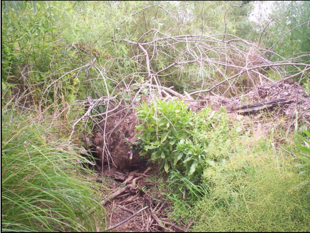
Photo 25. SPA 3. Debris jam caused by fallen tree at STA 32+50 – looking downstream.
