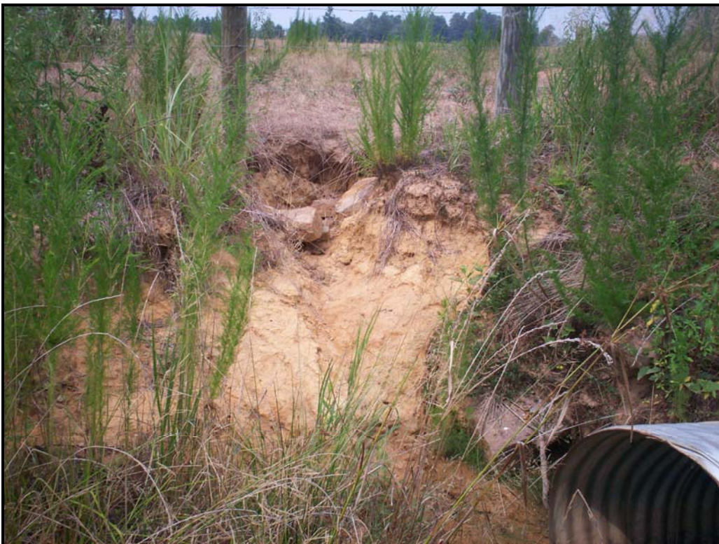
Photo 26. SPA 4. Left bank erosion at upstream end of culvert STA 30+60.
