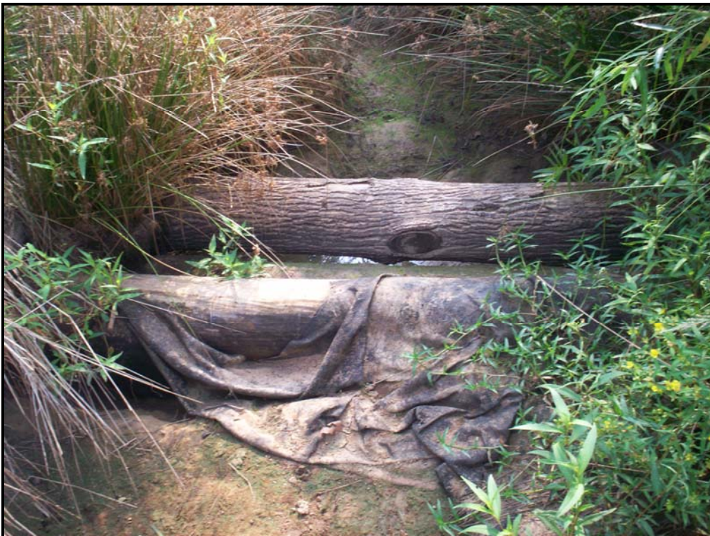
Photo 28. SPA 6. Grade control structure at STA 21+60-looking upstream; structure is not performing properly and has formed a head cut behind the structure.
