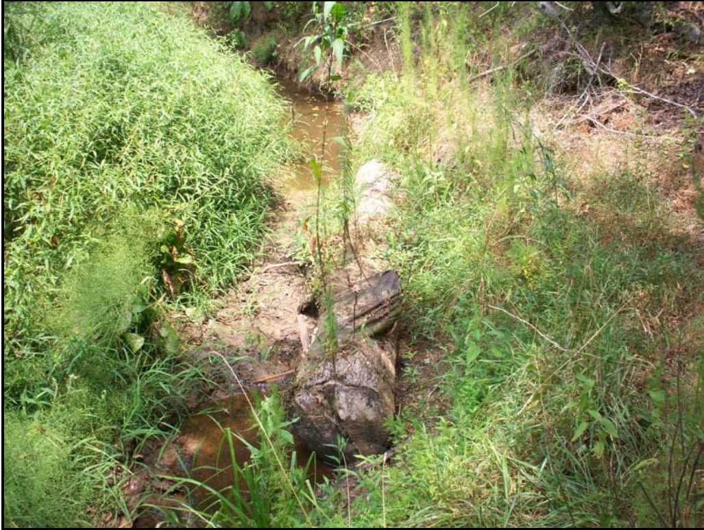
Photo 23. SPA 1. Log toe on right bank at STA 56+25; rolled into channel.
