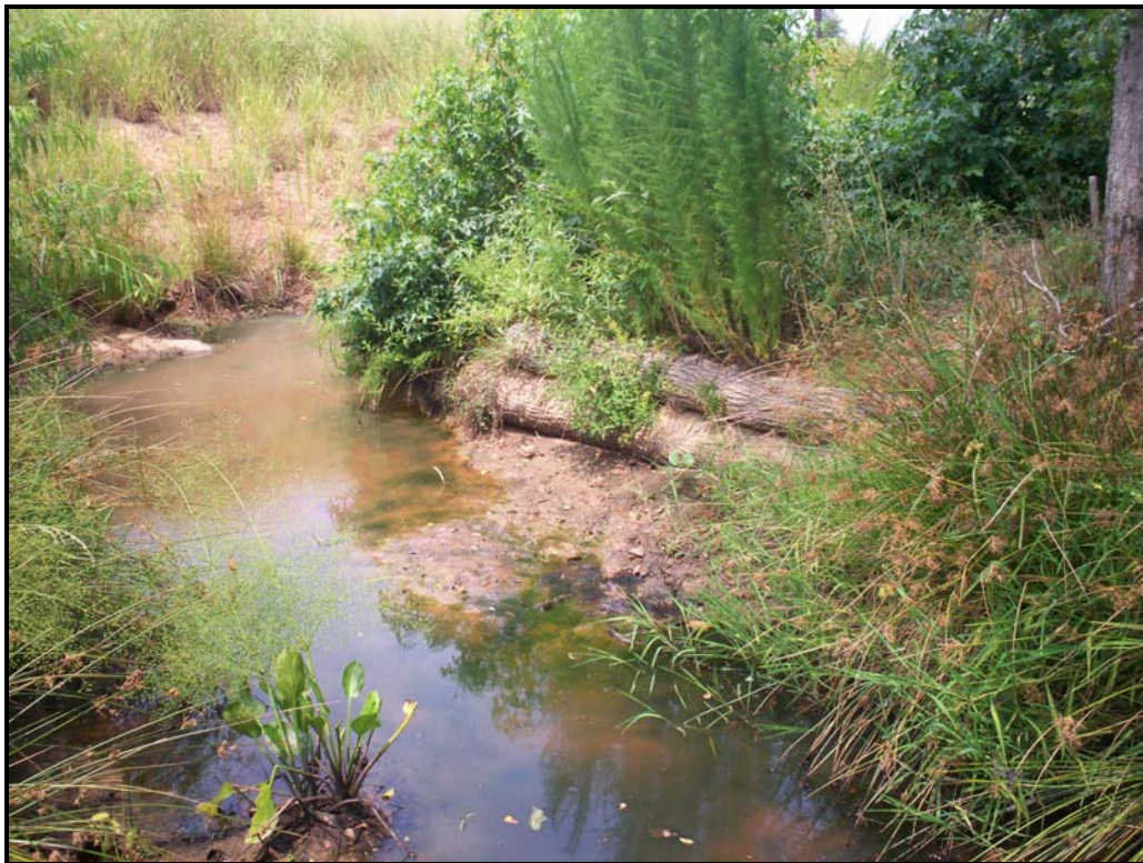
Photo 4. Log Toe at station 49+10 –looking downstream.
