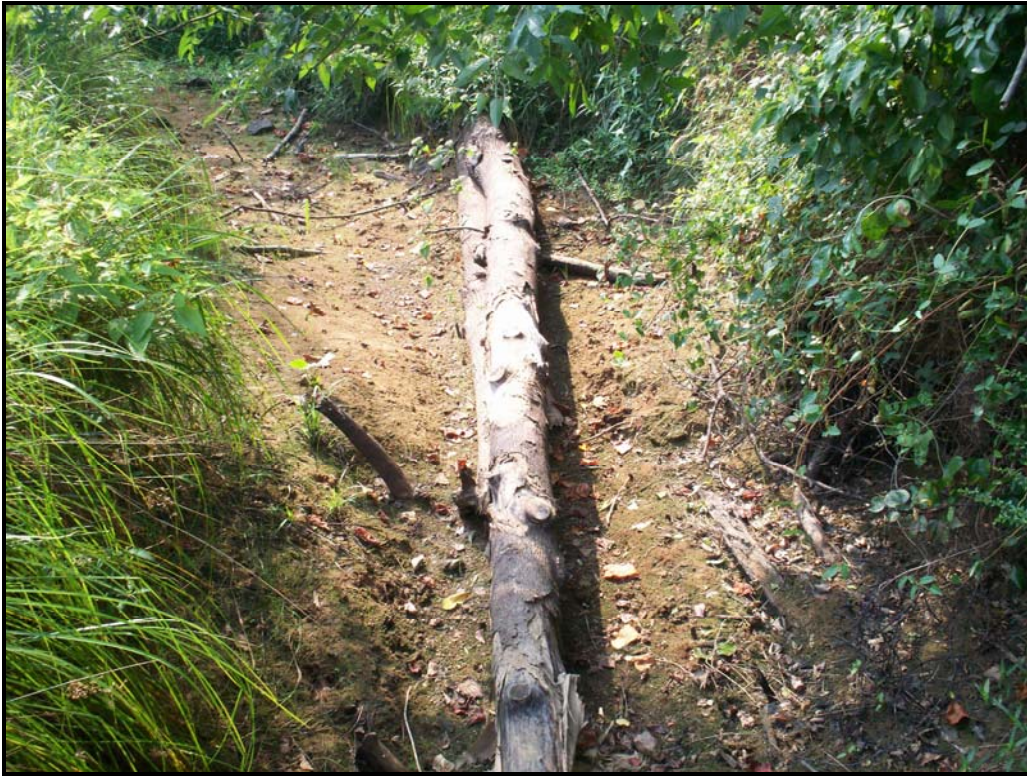
Photo 29. SPA 7. Log vane at STA 13+75 -looking downstream; US end of log vane is exposed.
