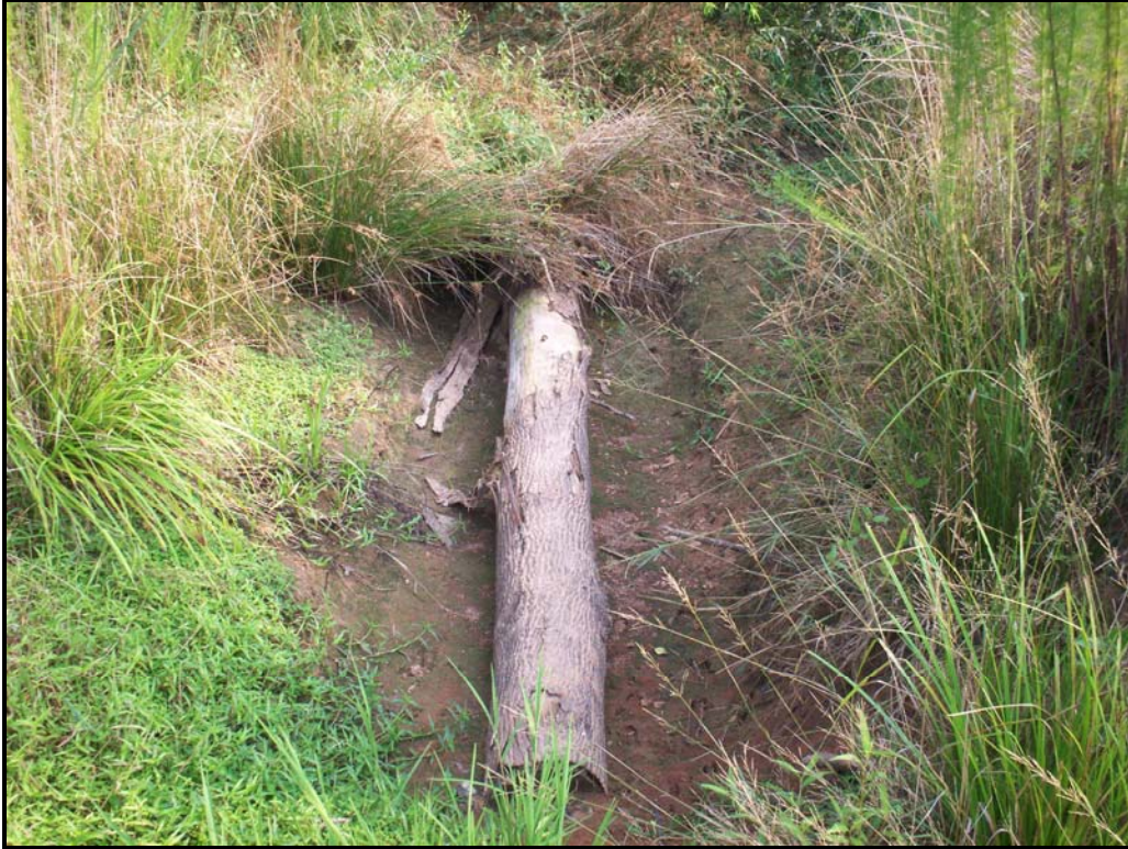
Photo 27. SPA 5. Log vane at STA 24+85-looking downstream; US end of log vane is exposed.
