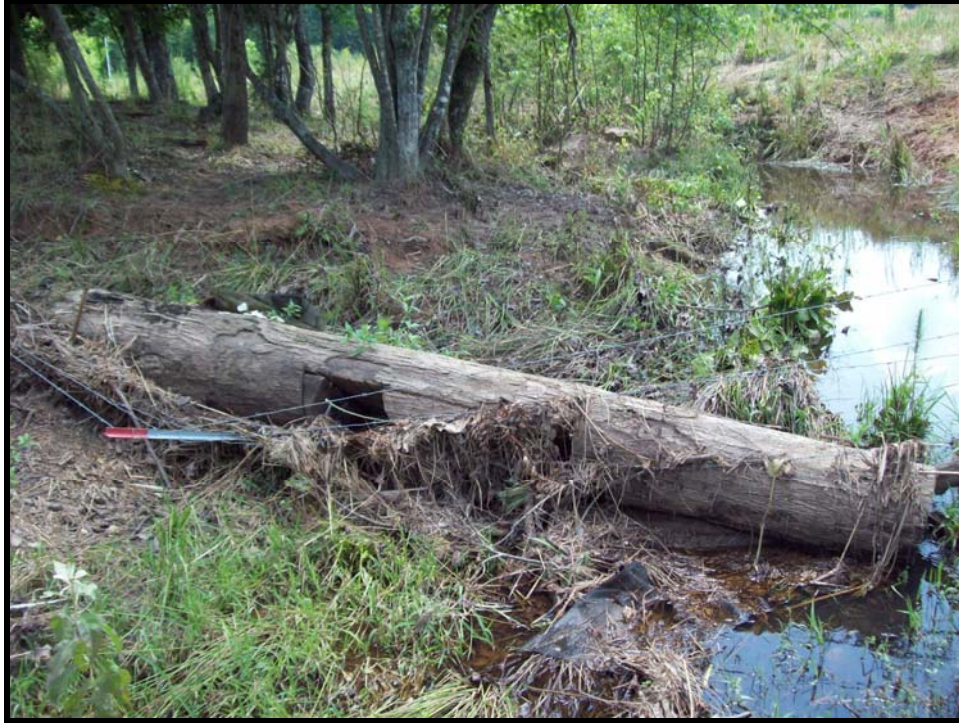
SPA 7. Fence knocked over by displaced log toe structure at Station 48+50.
