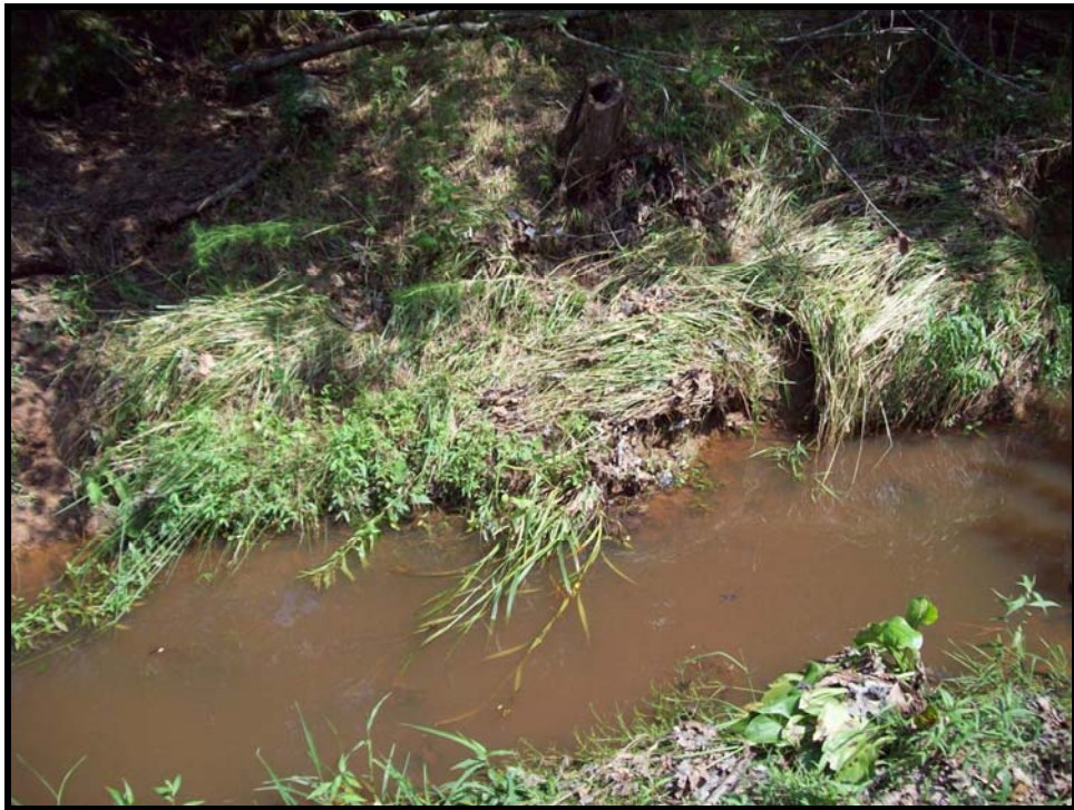
SPA 13. Log toe structure missing at Station 56+25.
