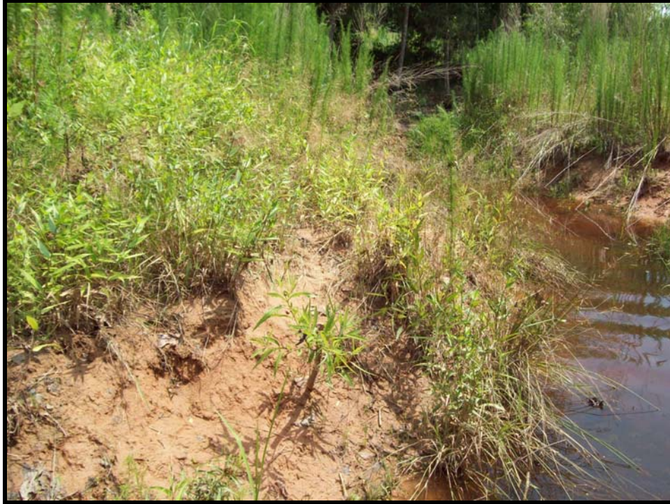
SPA 5. Minor erosion on right bank at Station 46+65.
