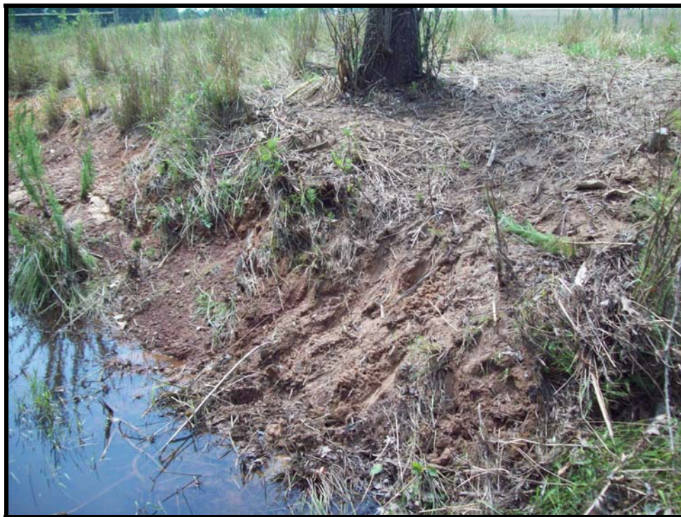
SPA 9. Erosion on left bank due to hoof shear from cattle at Station 48+60.
