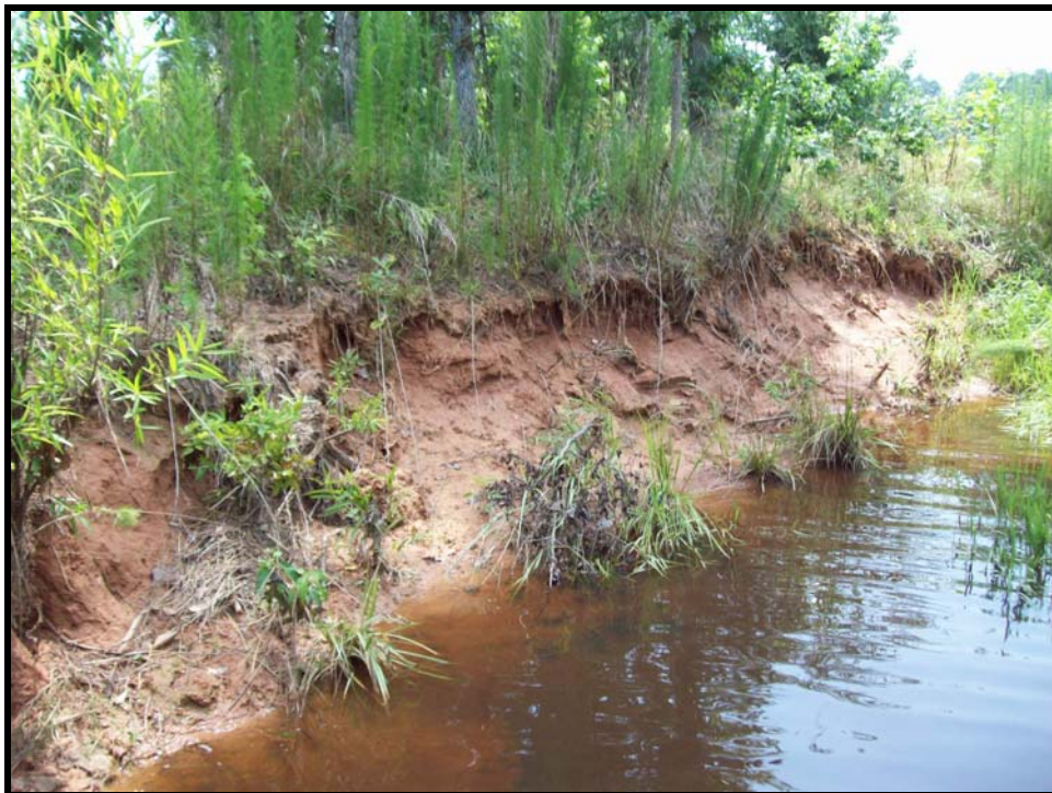
SPA 6. Erosion on right bank at Station 47+50.
