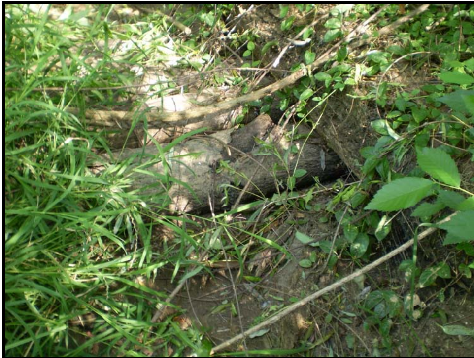
SPA 6 – Log grade control erosion, UT2, Sta. 2+50.
