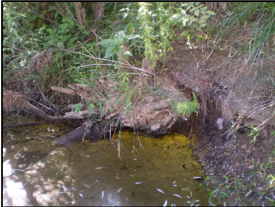
SPA 8 – Erosion behind root wad, UT1 Sta. 29+30.
