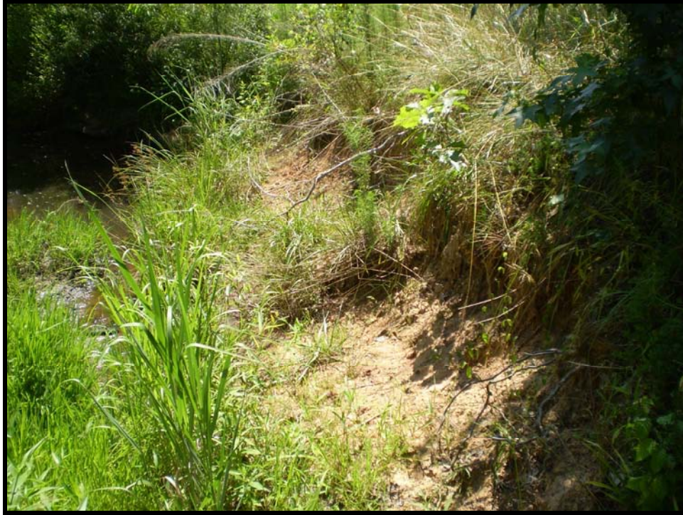
SPA 3 – Minor right bank erosion, UT1 Sta. 47+50 to 47+80.
