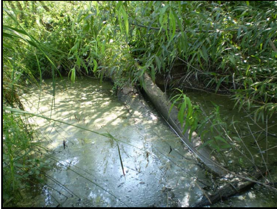
SPA 9 – Erosion behind log vane arm, UT1 Sta. 29+20.
