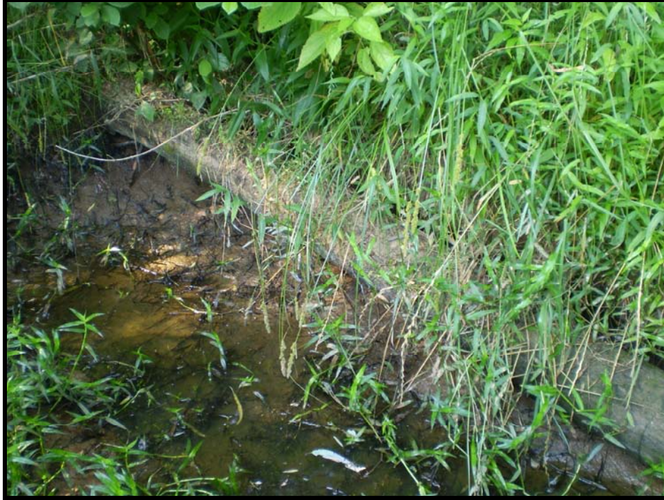
SPA 7 – Log vane erosion, UT1, Sta. 29+50.
