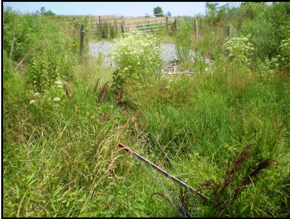
SPA 2 – Damaged fence, UT1 Sta. 48+00.
