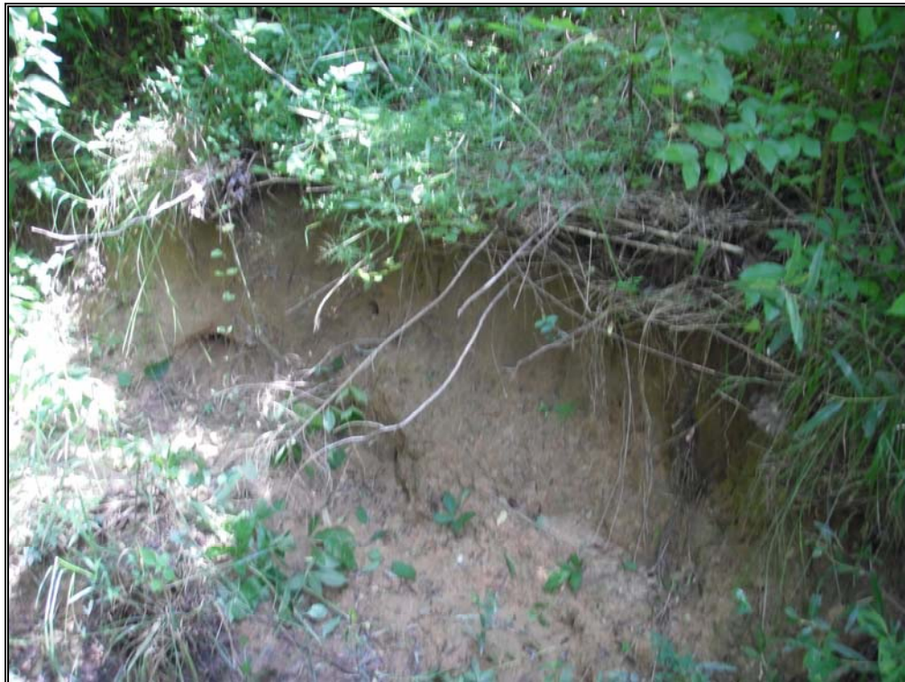
SOA 3 – Minor right bank erosion, UT1 Sta. 40+15 to 45+10.
