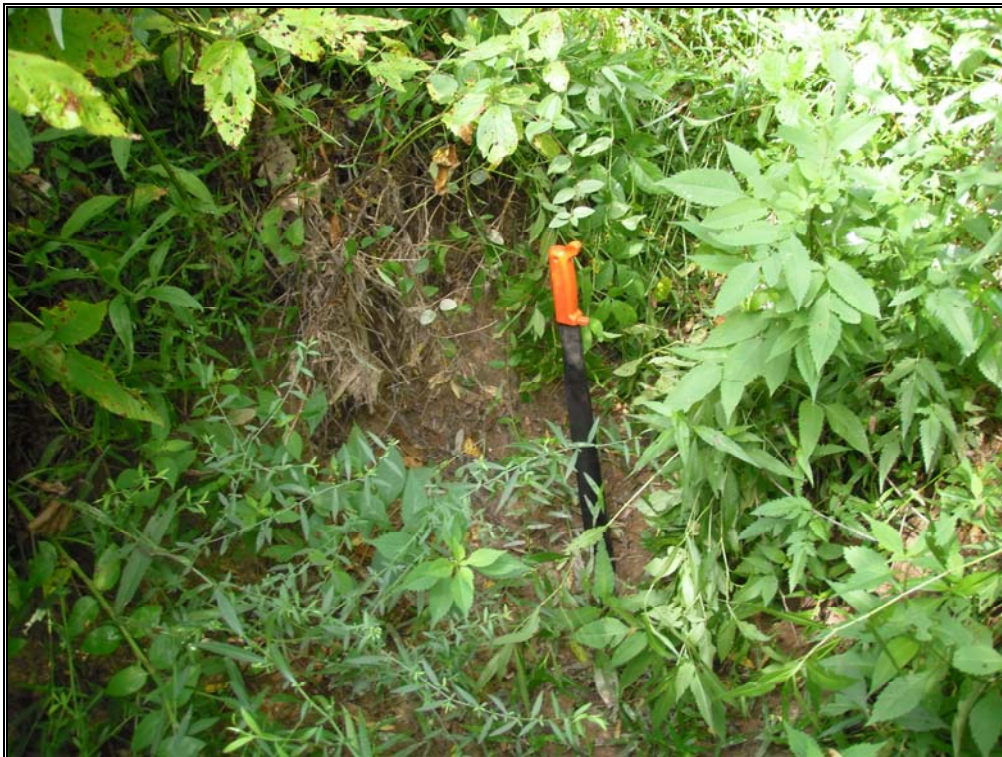
SOA 7 – Minor headcut. Vegetation has stabilized the channel., UT1 Sta. 2+15.
