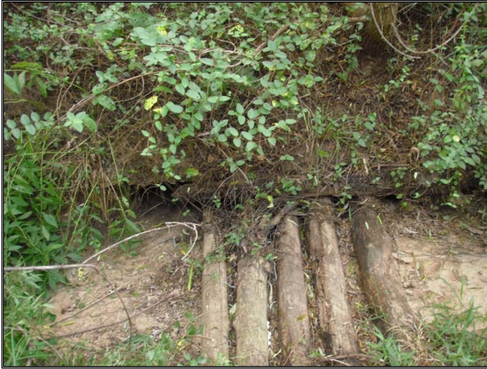
SOA 4 – Bank undercut along right bank at log grade control, UT2 Sta. 2+50.
