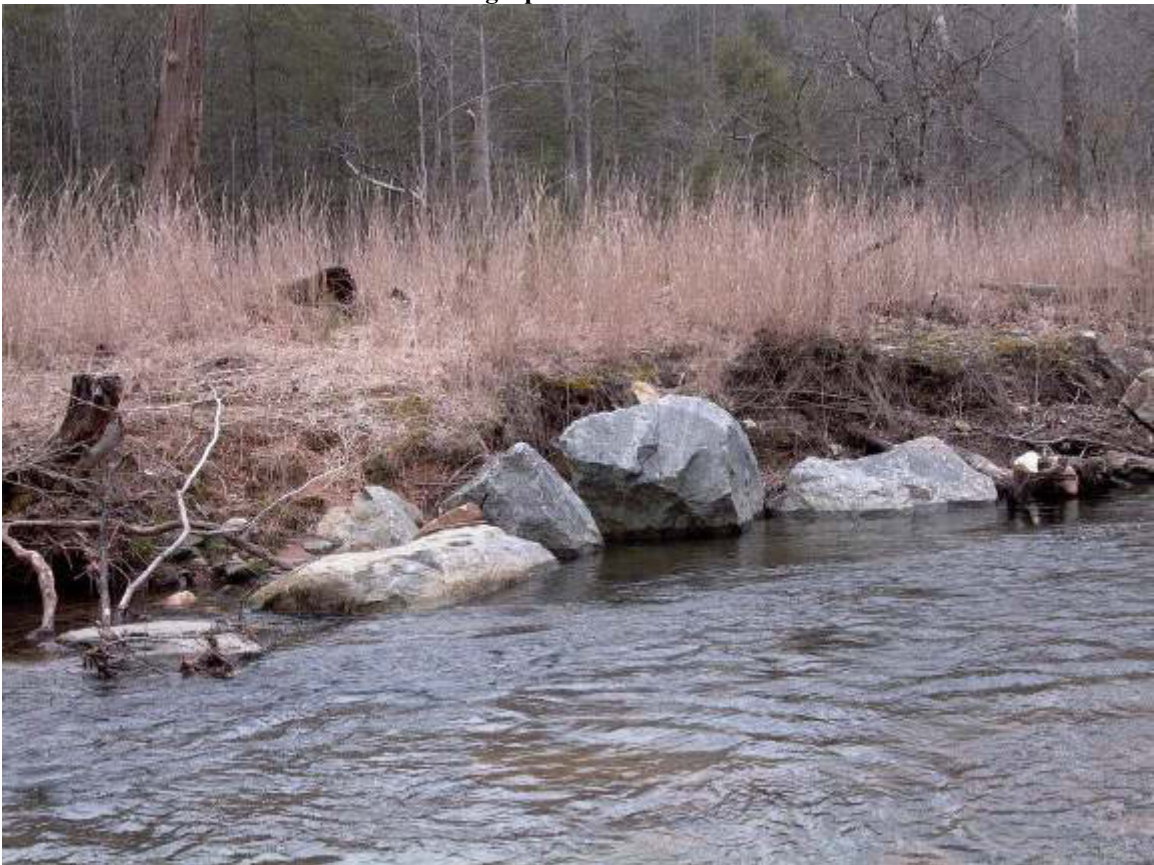
Looking Downstream at Left Bank Scour near J-Hook STA ~3+10
