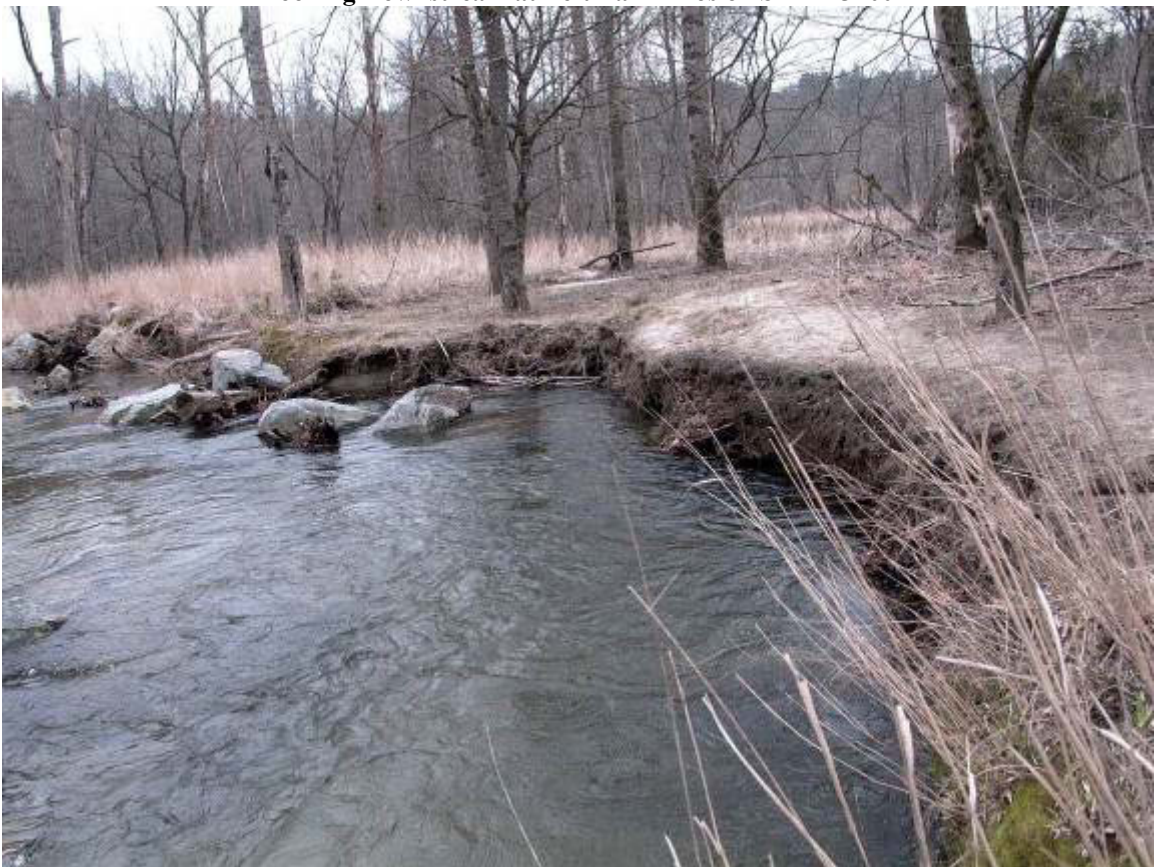
Looking Downstream at Right Bank Erosion and Migration STA ~ 5+60
