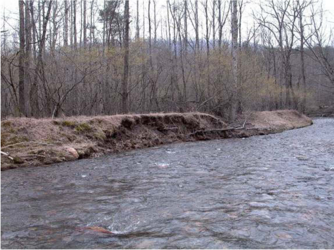
Looking Downstream at Left Bank Erosion STA ~ 3+00
