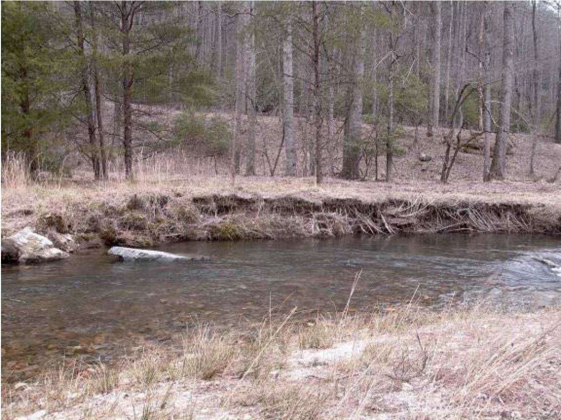
Looking Downstream at Left Bank Erosion and Migration STA ~ 8+50
