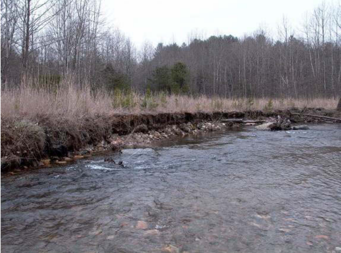
Looking Downstream at Left Bank Erosion and Migration STA ~ 28+75
