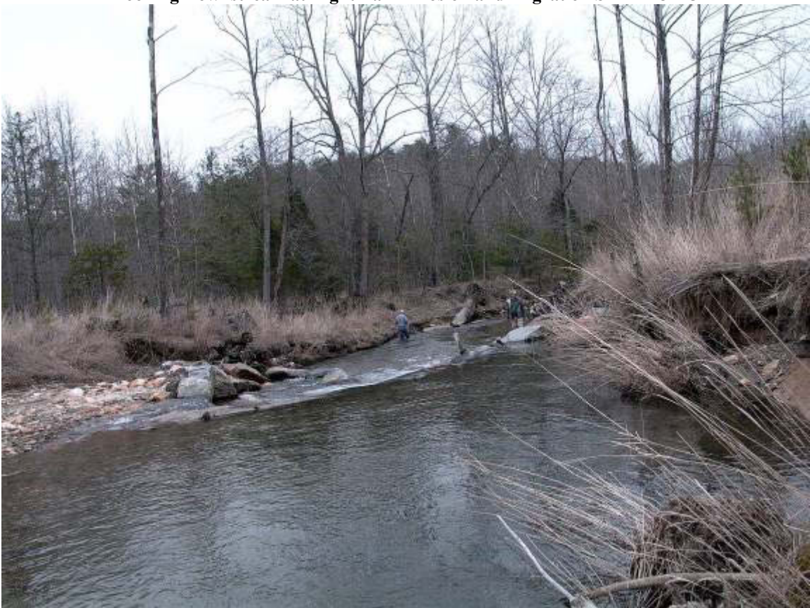
Looking Downstream at Right Bank Erosion & Piping Water around Rock Cross Vane STA ~ 24+40
