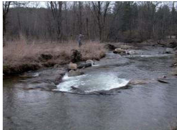
Issue Photo 2. Erosion Cross Vane STA ~12+90 Reach 4
