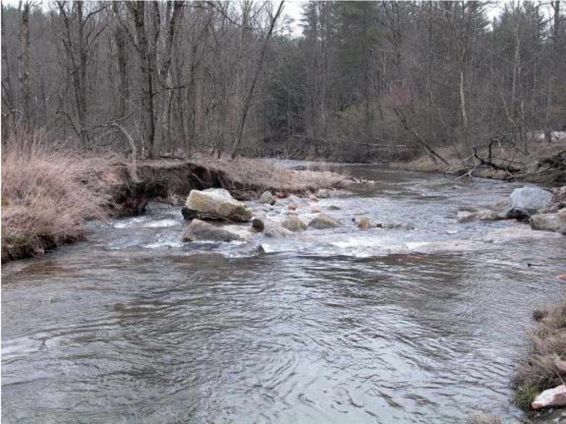
Looking Downstream at Left Bank Erosion & Piping Water Around Rock Cross Vane STA ~ 13+80
