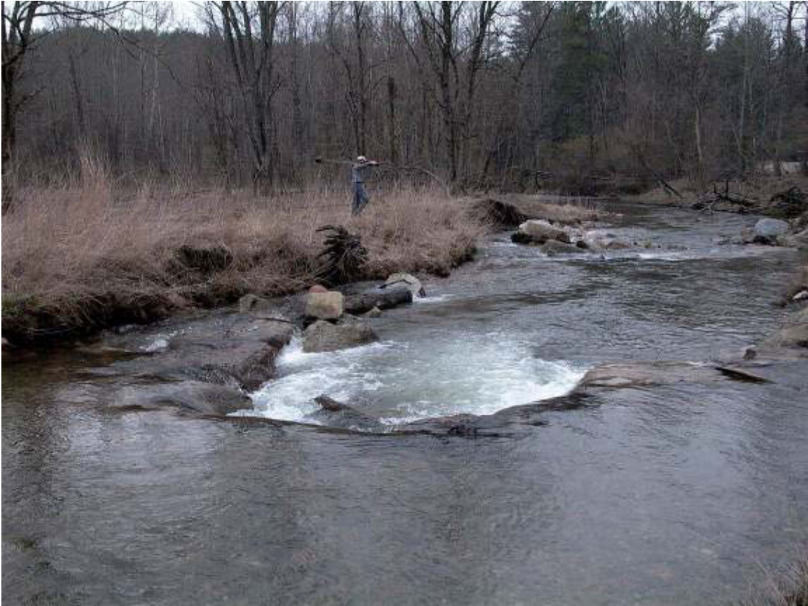
Looking Downstream at Left Bank Erosion & Piping Water Around Rock Cross Vane STA ~ 12+90
