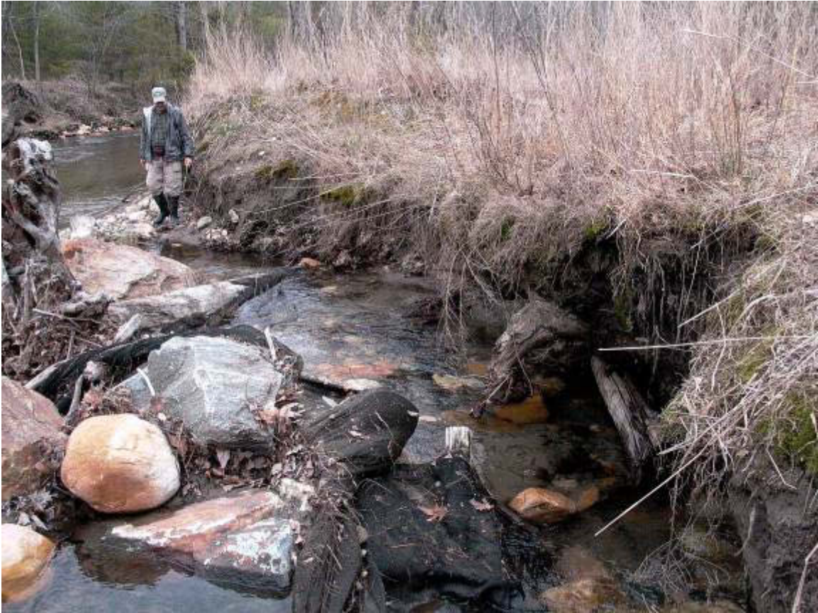
Looking Downstream at Right Bank Erosion & Piping Water around Rock Cross Vane STA ~ 24+80
