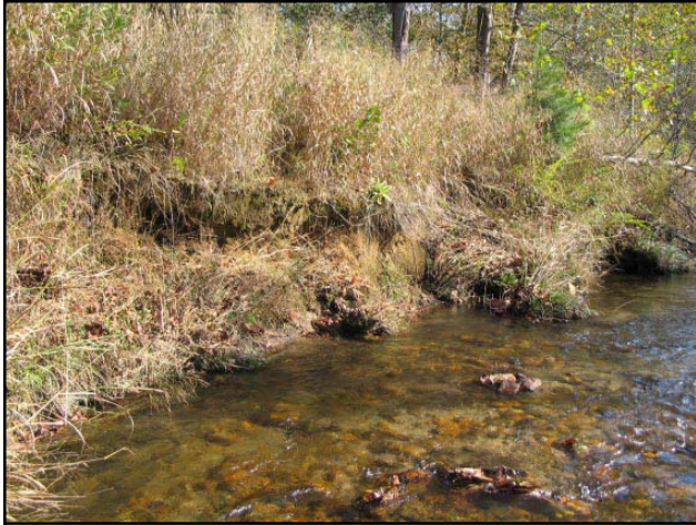
PA 21 Left Bank Erosion STA 19+00
