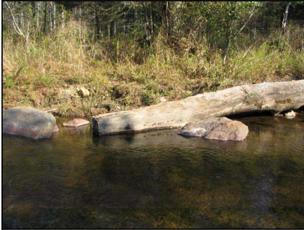
PA 30 Failed Log Vane Left Bank 26+00
