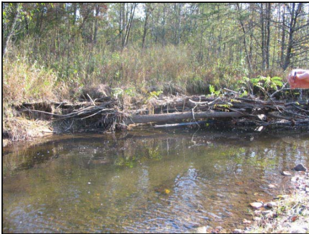
PA 22 Looking Downstream STA 20+25 Left Bank Erosion
