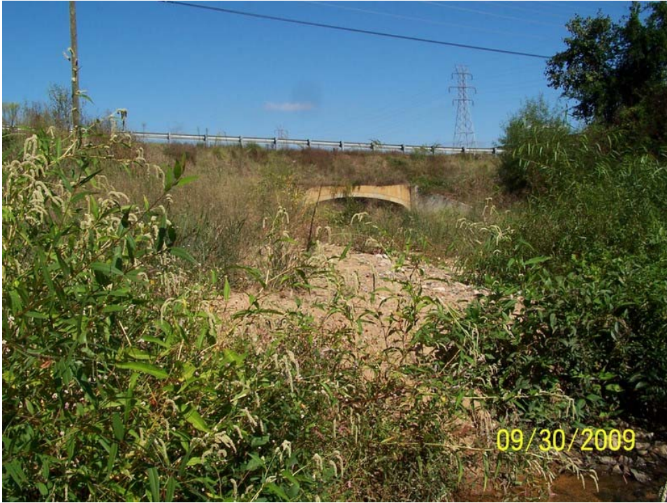
Sand deposition below bridge at Sign Drive
