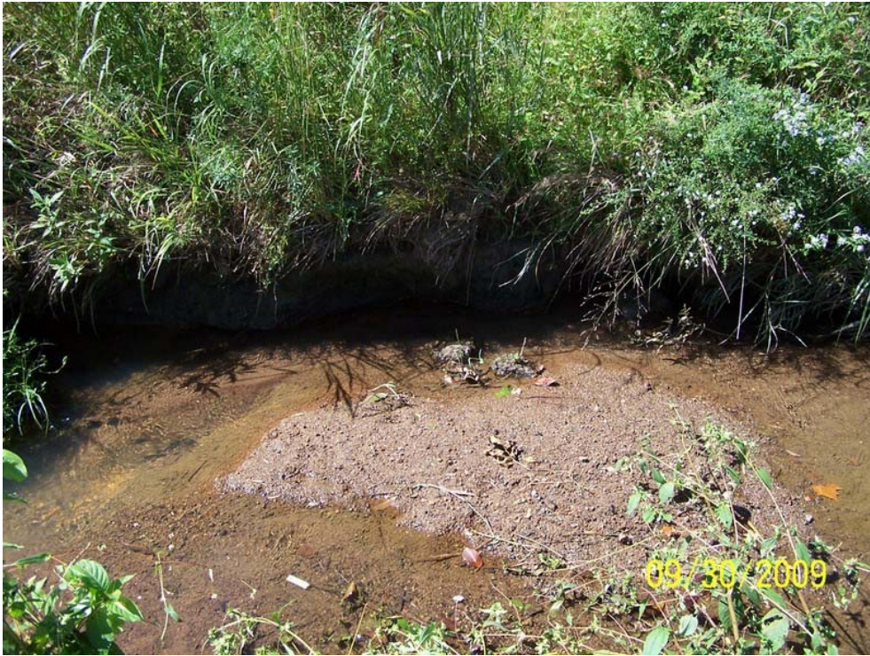
Small problem area just downstream of XS 1, will be live staked and watched
