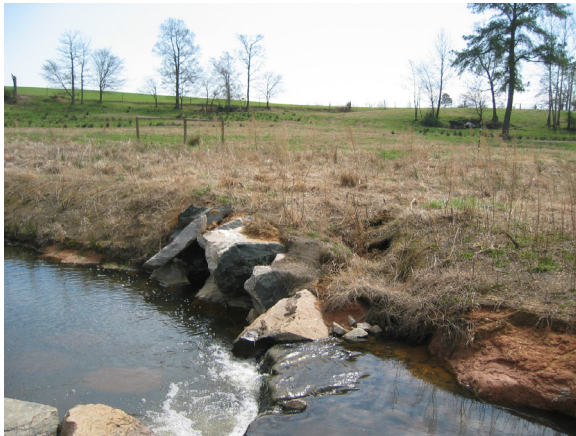
Photo 6: Structure Arm Scour - Station 17+50
