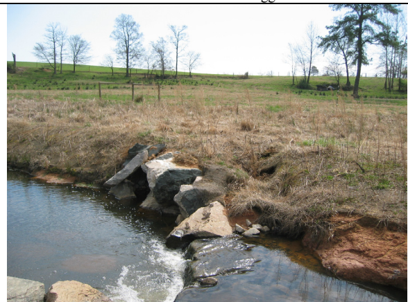
Photo 6: Issue 3 - Structure Arm Scour
