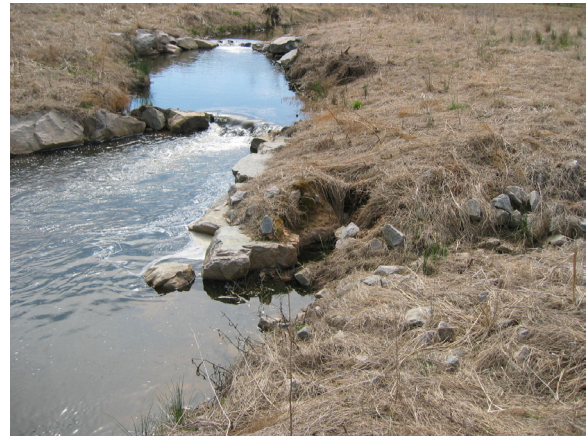
Photo 7: Structure Arm Scour - Station 18+00
