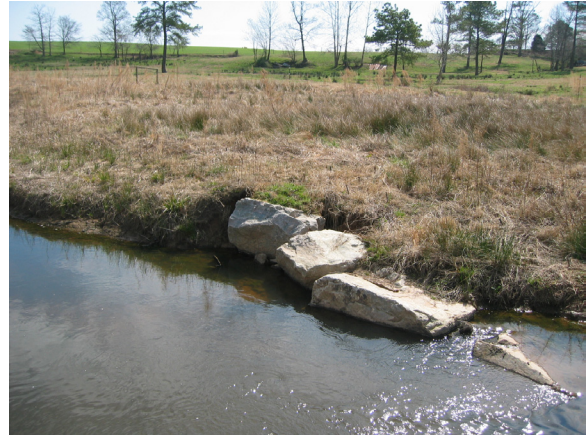
Photo 5: Structure Arm Scour - Station 16+00
