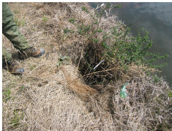
Photo 2: Evidence of Bank Erosion - Station 13+50
