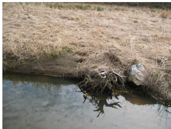
Photo 4: Evidence of Bank Erosion - Station 21+00
