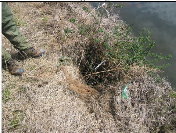
Photo 5: Issue 2 - Bank Erosion
