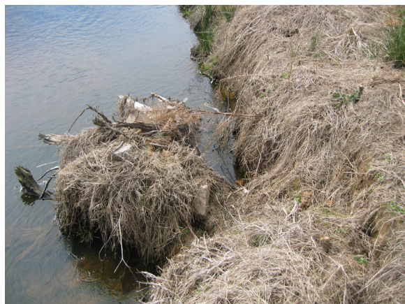
Photo 3: Evidence of Bank Erosion - Station 18+25
