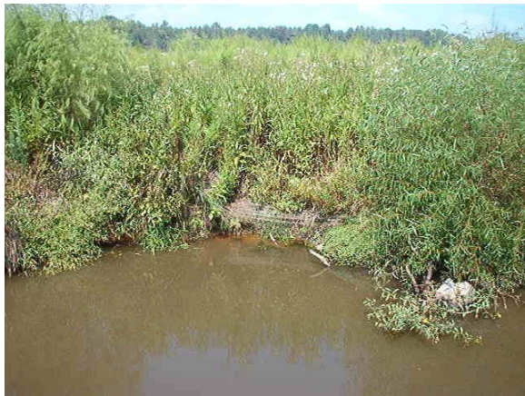
Photo 14, bank scour at station 11+50
