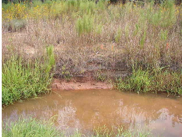
Photo 7, bank scour and un-vegetated floodplain bench at station 22+80.
