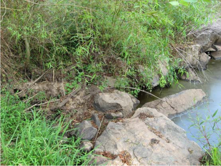
Station 26+60, left bank arm scour
