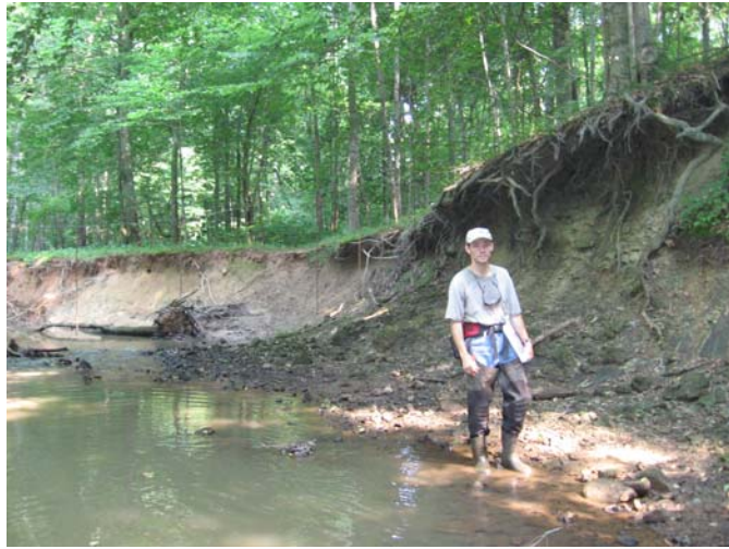
1. Main Channel Bank Erosion 7.26.2006
