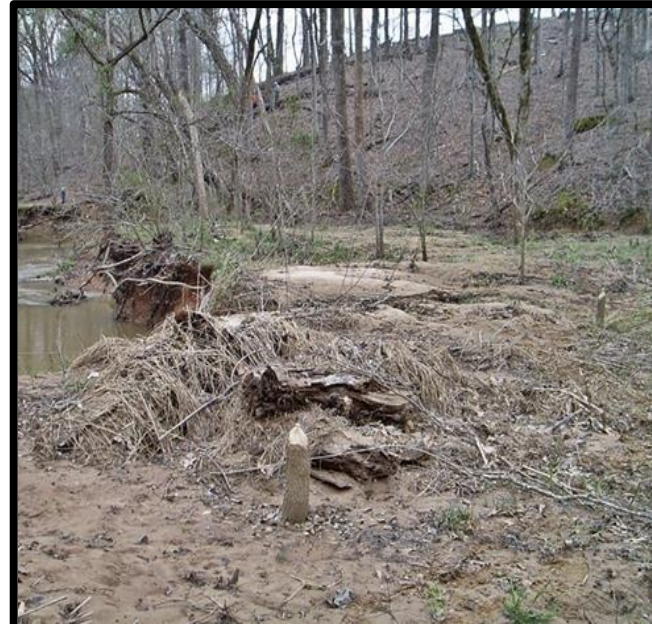
Vegetation Problem Area 2: Beaver-cut trees and low stem density along DBC right bank, station 16+50. 10Apr2014.
