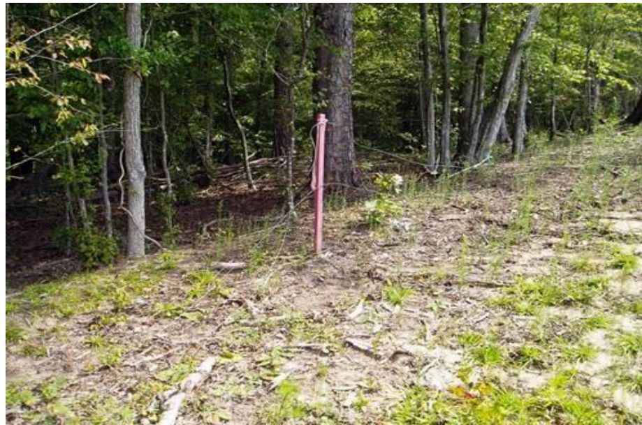
Easement fence broken, SE of PhoPt-2, DBC sta 15+00, Sep 2015
