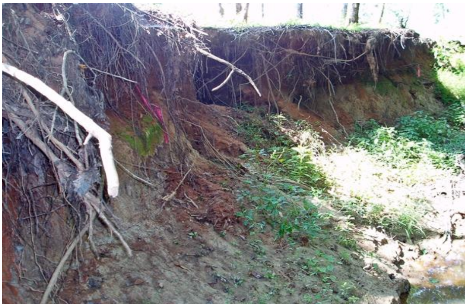
DBC RBK sta 28+30 erosion pins 6-7, face upst, Sep 2015
