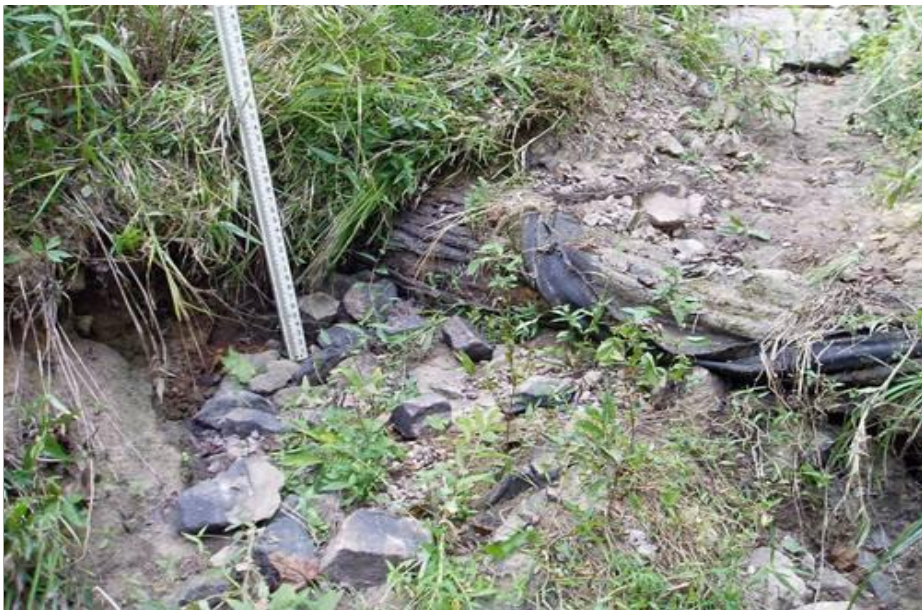
Bank erosion at step-pool: Tributary station 5+30, Sep 2015
