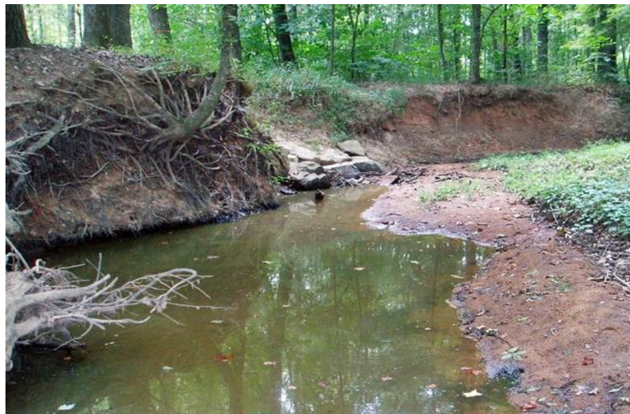
DBC sta 35+80, face upst, RBK erosion, Sep 2015
