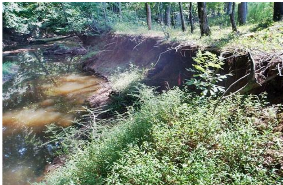
DBC RBK sta 28+30 erosion pins 6-7, face dnst, Sep 2015
