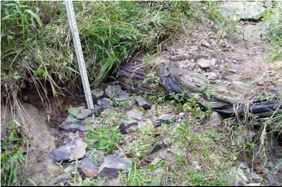
Bank erosion at step-pool: Tributary station 5+30, Sept 2015
