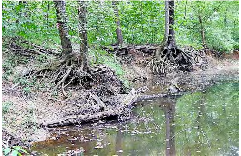
Bank Erosion: Tributary Station 23+50, Sept 2016
