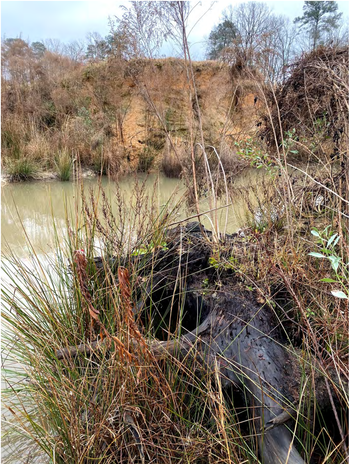
Photo 2.) UT-2 Failed Crossing – Historic floodplain elevation with historic tree roots visible at break between historic floodplain and fill material
