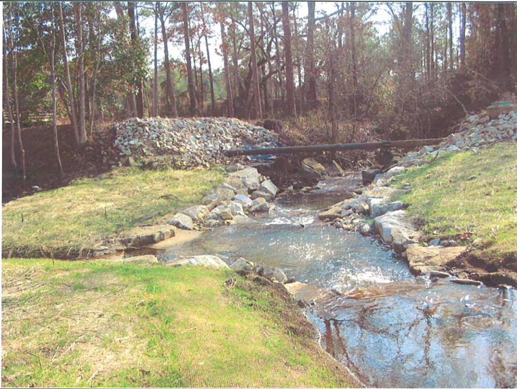
Photograph 5. Phase I Completed: Southeast view of restored stream at utility crossing. Photo taken 1/12/2006.
