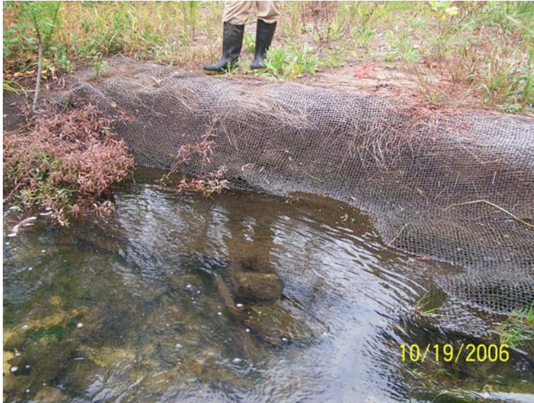
Problem Area 1 – Rocks and bank under matting have settled. Vegetation hasn't taken root due to rock under matting, area will be live staked this winter.
