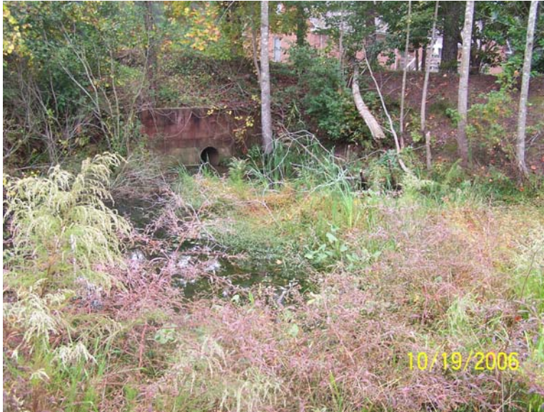
Photo Point 1 – Storm Water BMP
