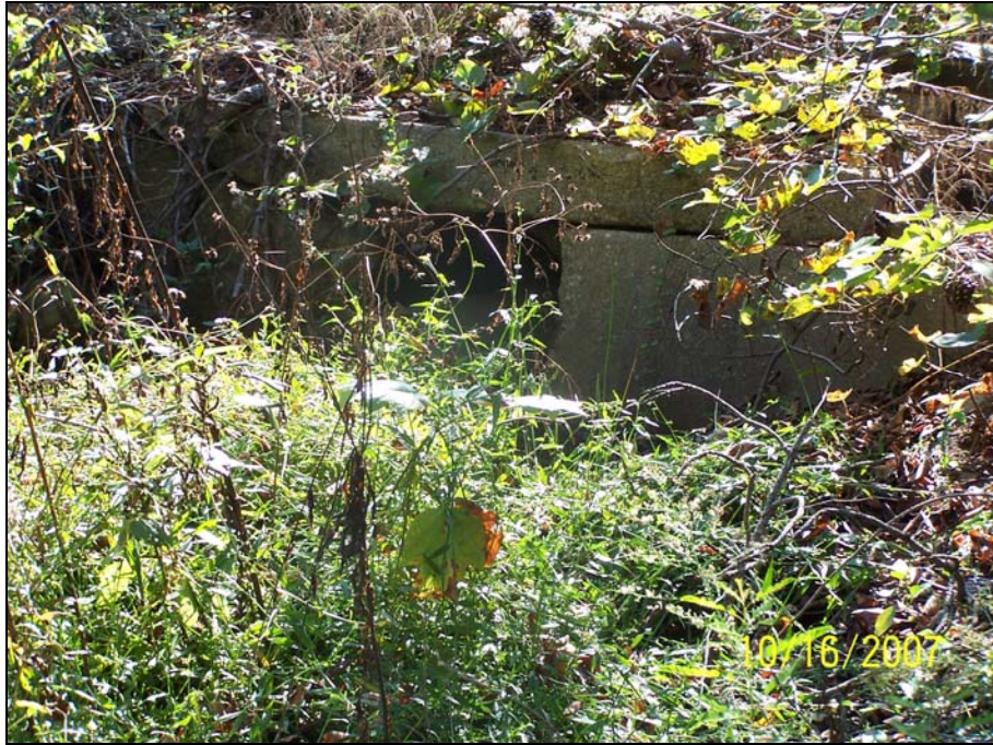
Storm water outfall 5, located in eastern prong in the stream restoration section.
