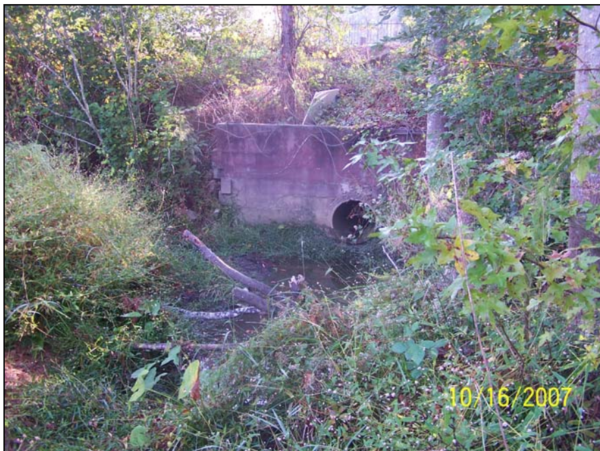
Storm water outfall 4, located in eastern prong in stream restoration section (near cross-section 1, also photo point 1).
