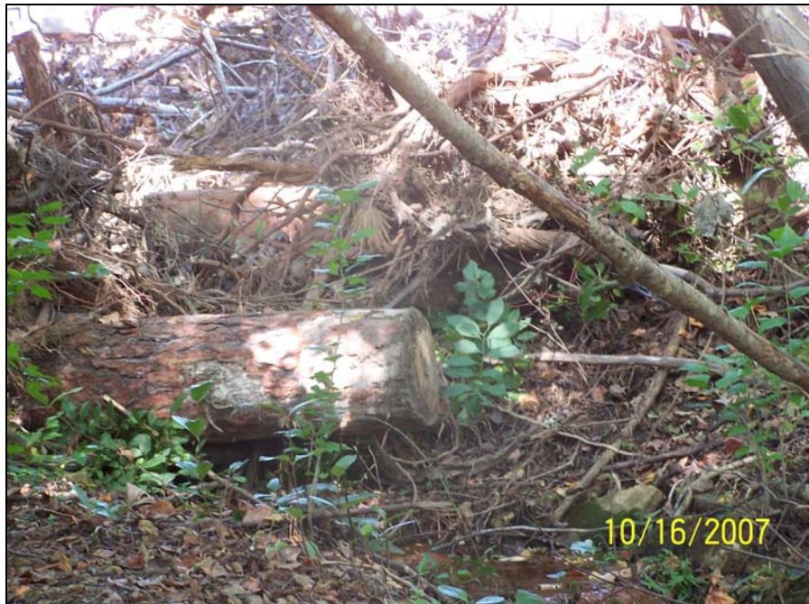
Storm water outfall 7 has debris blocking it from the landowner doing construction.
