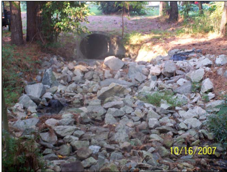
Storm water outfall 1, located in western prong in stream enhancement section (near well CE2).
