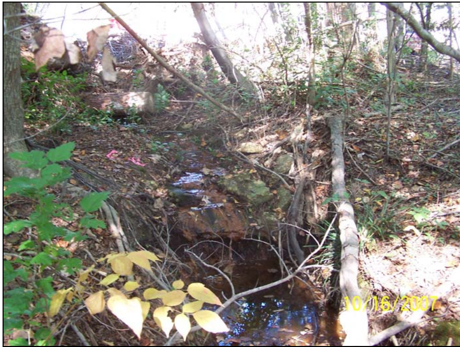
Storm water outfall 7, located in the eastern prong in the stream restoration section (near well CEC10).
