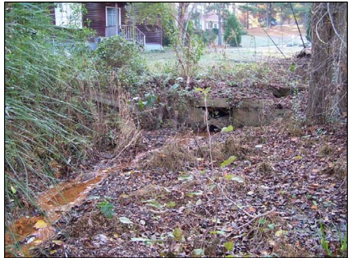
Outfall S of monitoring well CEC10
