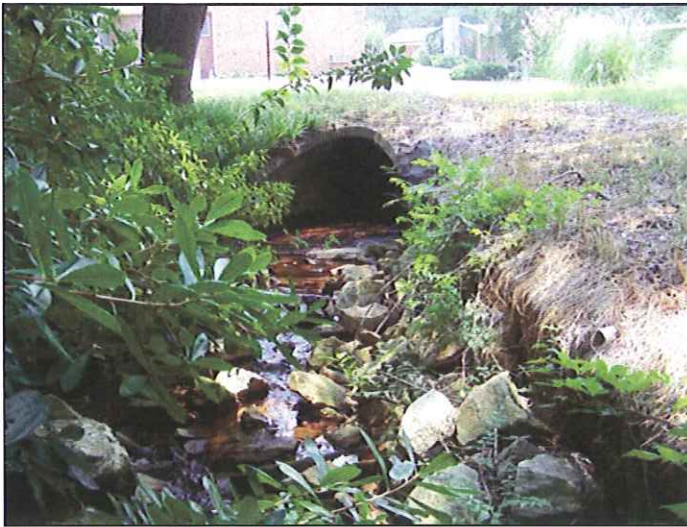
Outfall W of well TARLTON4
