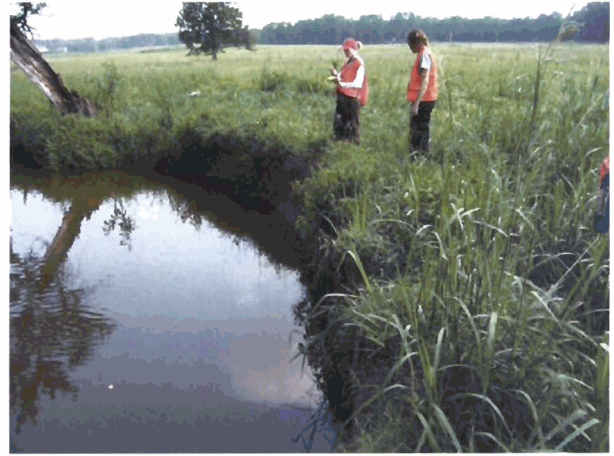
Outer Bend #8 - Looking Upstream (Severe Erosion)
