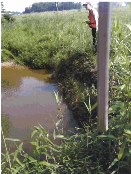
Outer Bend #16 - Looking Upstream at tight bends. This is not a good reach for bank stabilization comparisons. (Moderate Erosion)
