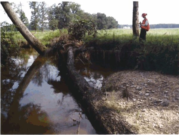
Outer Bend #12 - Looking Upstream (Severe Erosion)
