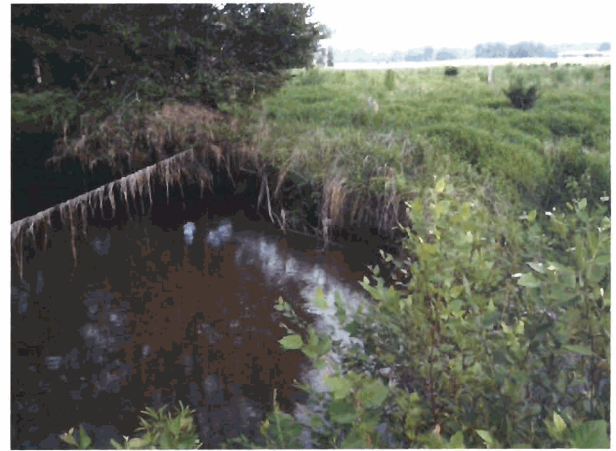
Outer Bend #12 - Looking Upstream (Severe Erosion)
