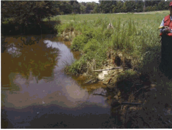
Outer Bend #27 - Looking Upstream at erosion on low slope reach. (Severe Erosion)
