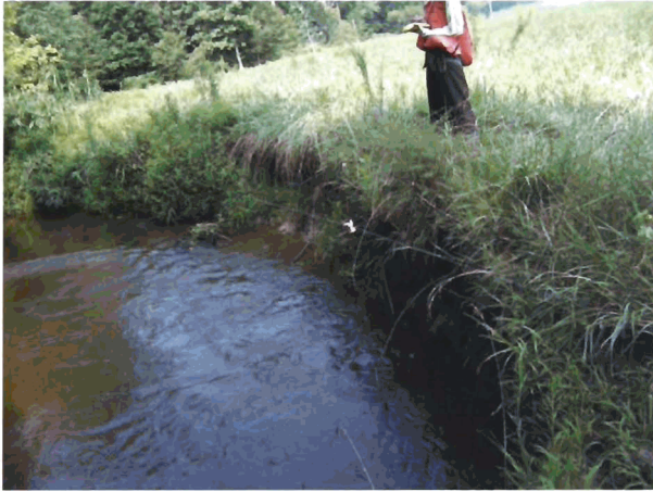
Outer Bend #14 - Looking Upstream at tight radius caused by point bar and transverse bar. (Severe Erosion)
