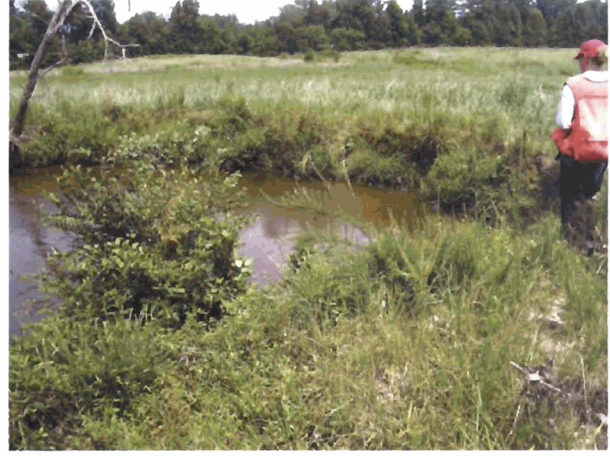
Outer Bend #28 - Looking Upstream at potential shoot cutoff development. (Severe Erosion)
