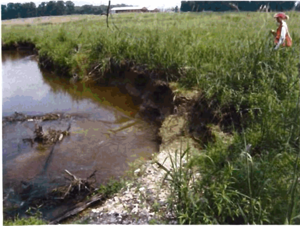
Outer Bend #18 - Looking Upstream (Extreme Erosion)
