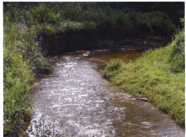
Outer Bend #20 - Looking Downstream at a long bend with a tight radius in the middle of the bend. (Extreme Erosion)
