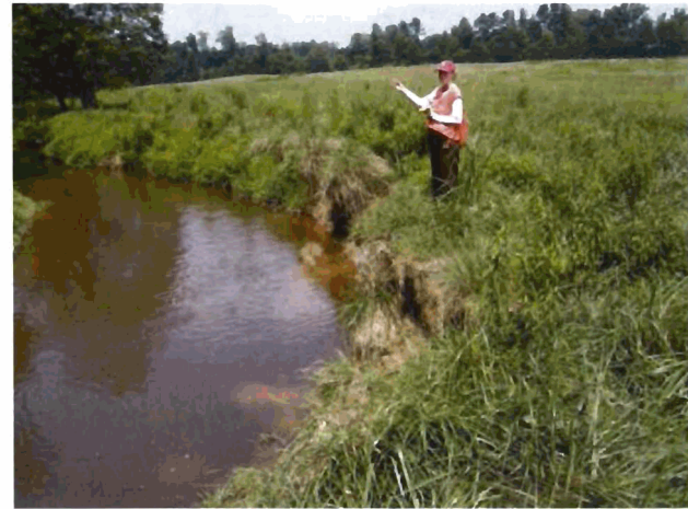
Outer Bend #24 - Looking Upstream at a short reach of erosion. (Severe Erosion)
