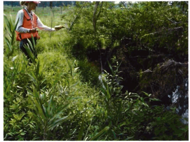
Outer Bend #17 - Looking Downstream (Severe Erosion)
