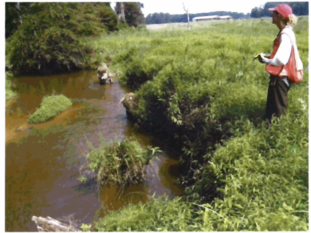
Outer Bend #15 - Looking Upstream at a long bend with two stumps extending into the stream. (Moderate Erosion)
