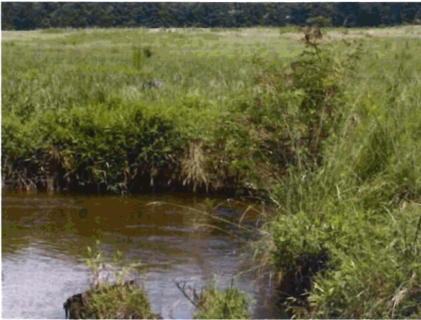
Outer Bend #23 - Looking Upstream at root balls in channel and bank sloughing (Severe Erosion)
