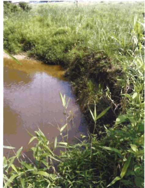
Outer Bend #16 - Looking Upstream at tight bends. This is not a good reach for bank stabilization comparisons. (Moderate Erosion)
