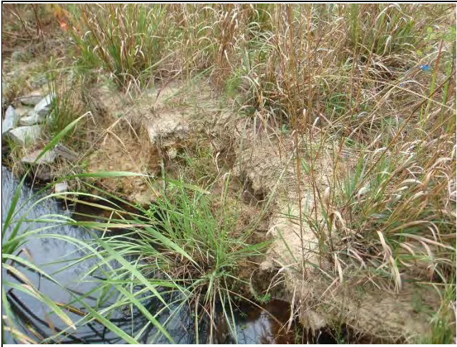
R2 bank scour MY3 (photo: 6/13/18)
