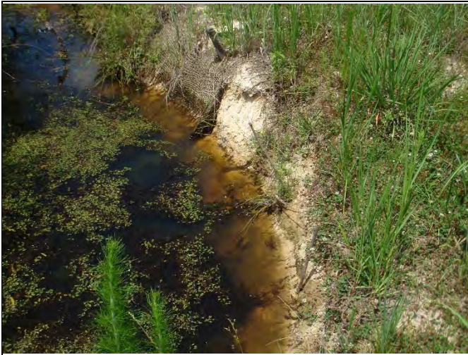
R2 bank scour MY3 (photo: 6/13/18)
