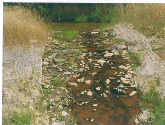
Photograph No. 4- Triple Log Sill at Station 11+95 on Unnamed Tributary, Looking Upstream
