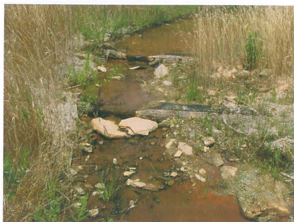
Photograph No. 3- Double Log Sill at Station 7+74 on Unnamed Tributary, Looking Upstream
