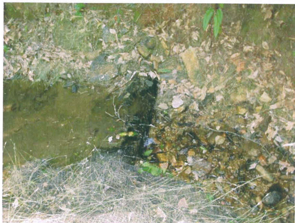
Photograph No. 1- Single Log Sill at Station 0+50 on Unnamed Tributary, Looking Across Stream
