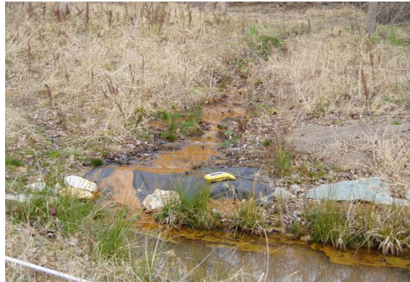
SP4. Exposed Matting
