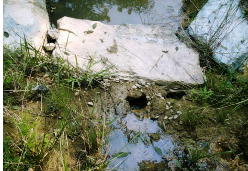
SP2. Piping and minor backcutting (hook/vane)
