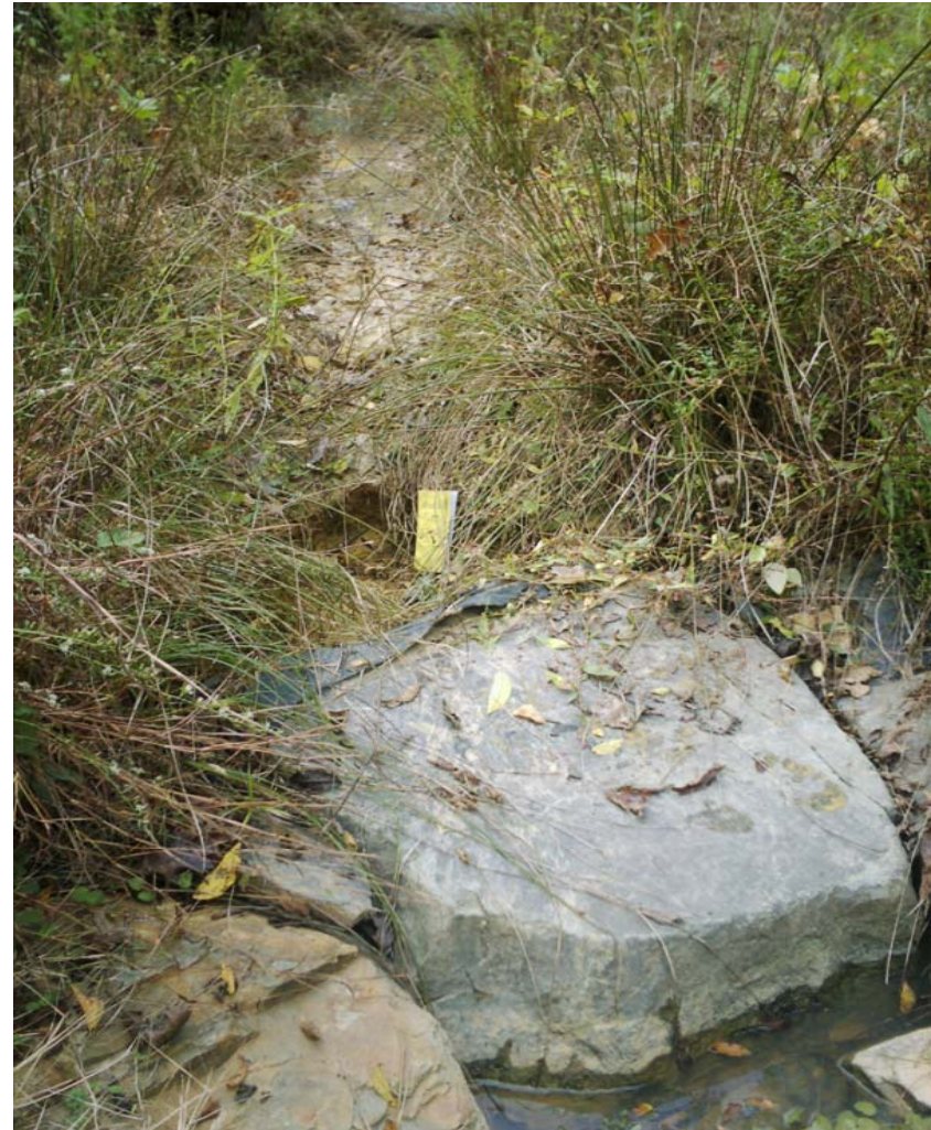
SP2. Piping and headcutting
