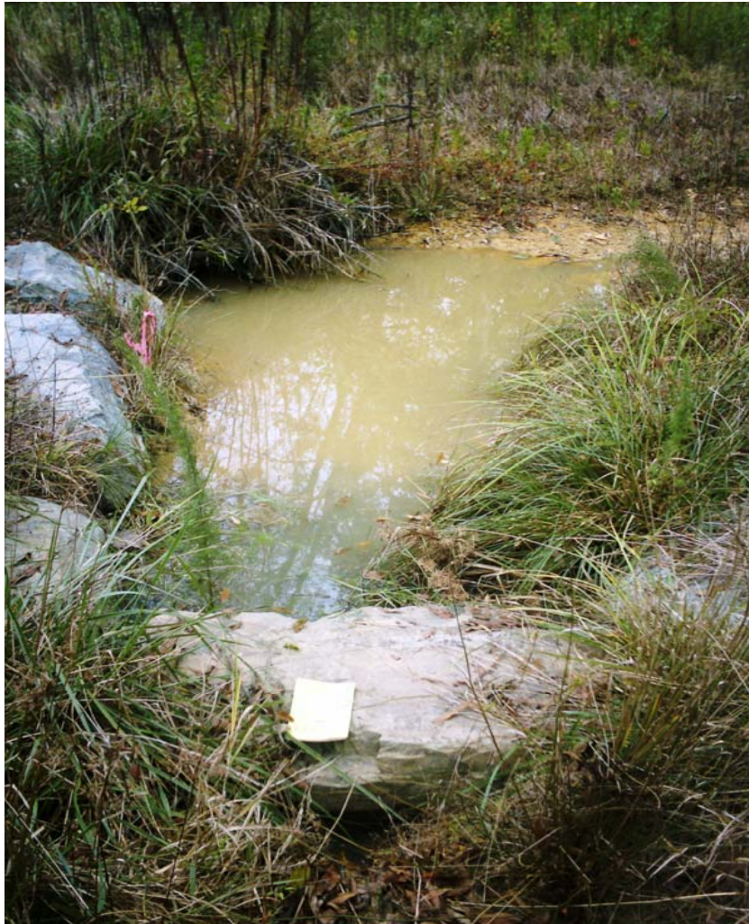
SP1. Piping above rock structure
