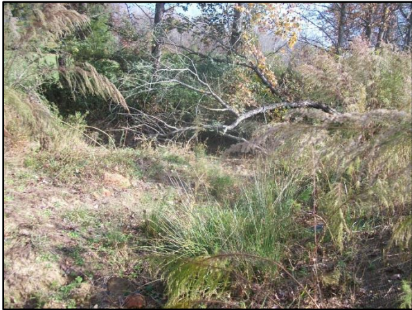
PID 43: Station 48+05 – Downstream (11/06/17)
