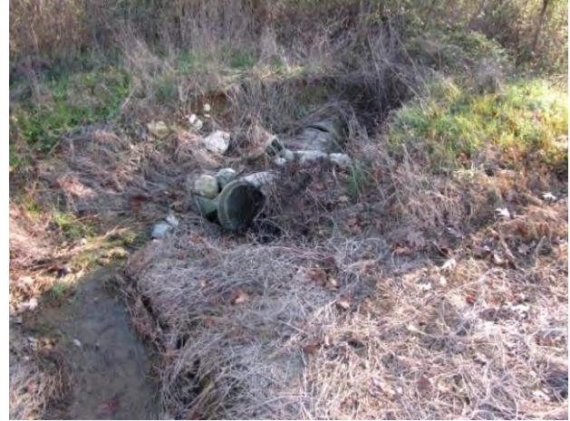
Photo 8: View of damaged culvert separating Tributary 1A and 1B: December 2011
