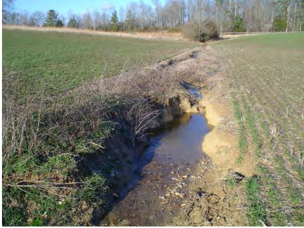
Photo 1: Headcut on upper portion of Tributary 1A: February 2010
