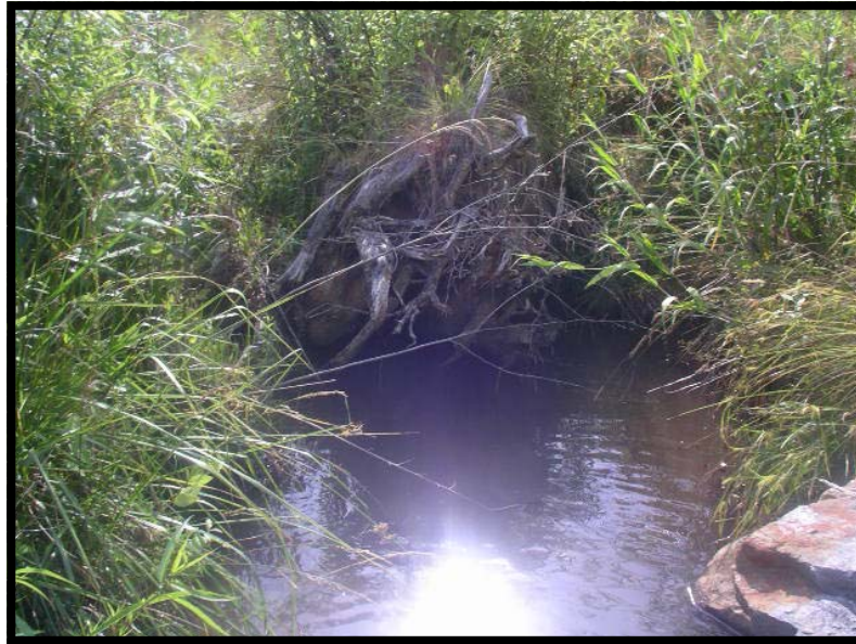
Figure 5—Typical Bank Scour
