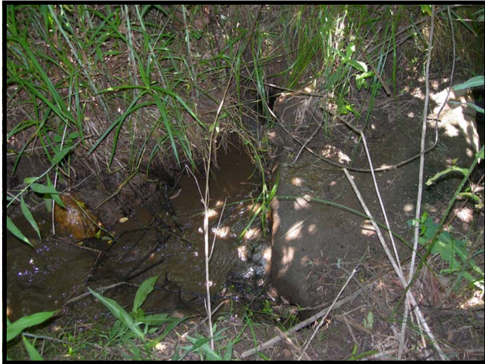
Figure 3—Typical Rock Piping (June 12, 2007)
