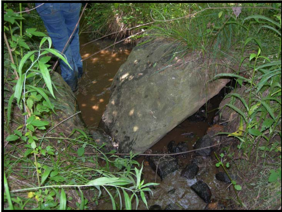
Figure 1—Typical Rock Shift (June 12, 2007)
