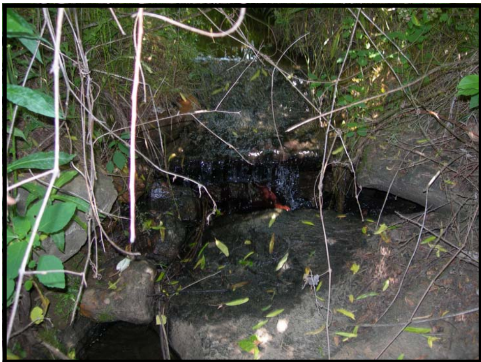
Figure 2—Typical Rock Shift (June 12, 2007)
