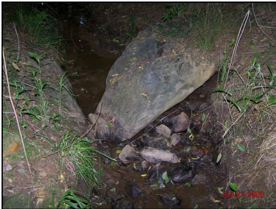
Stream Problem Area (SPA 2) – Failed structure Monitoring Year 4 – June 27, 2008
