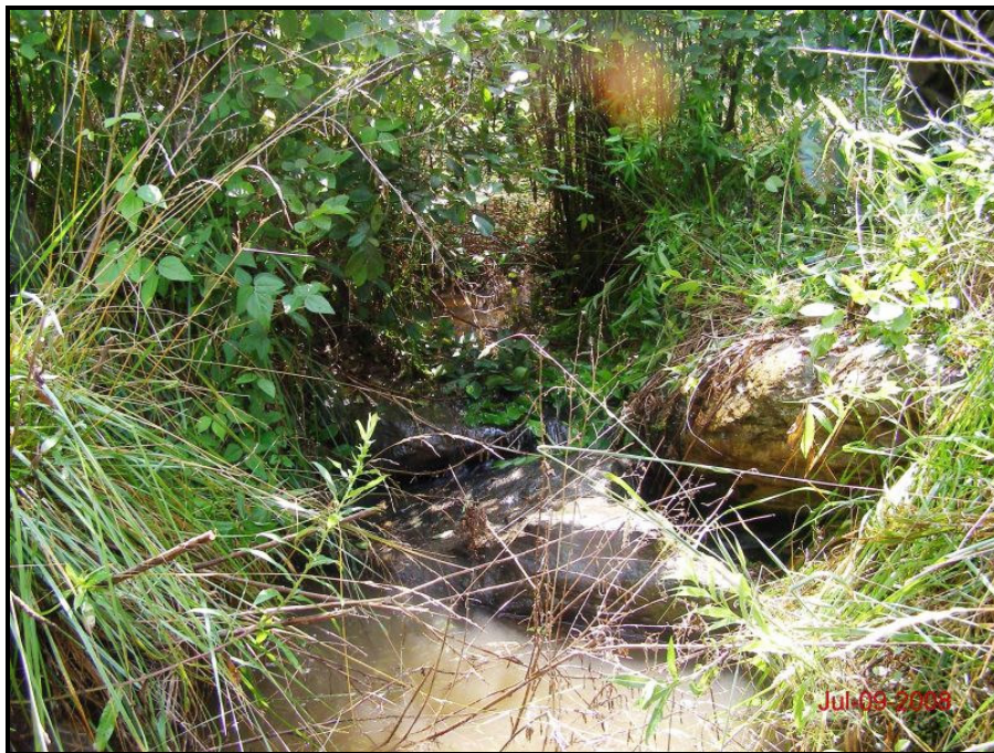
Stream Problem Area (SPA 4) – Stressed structure Monitoring Year 4 – July 9, 2008
