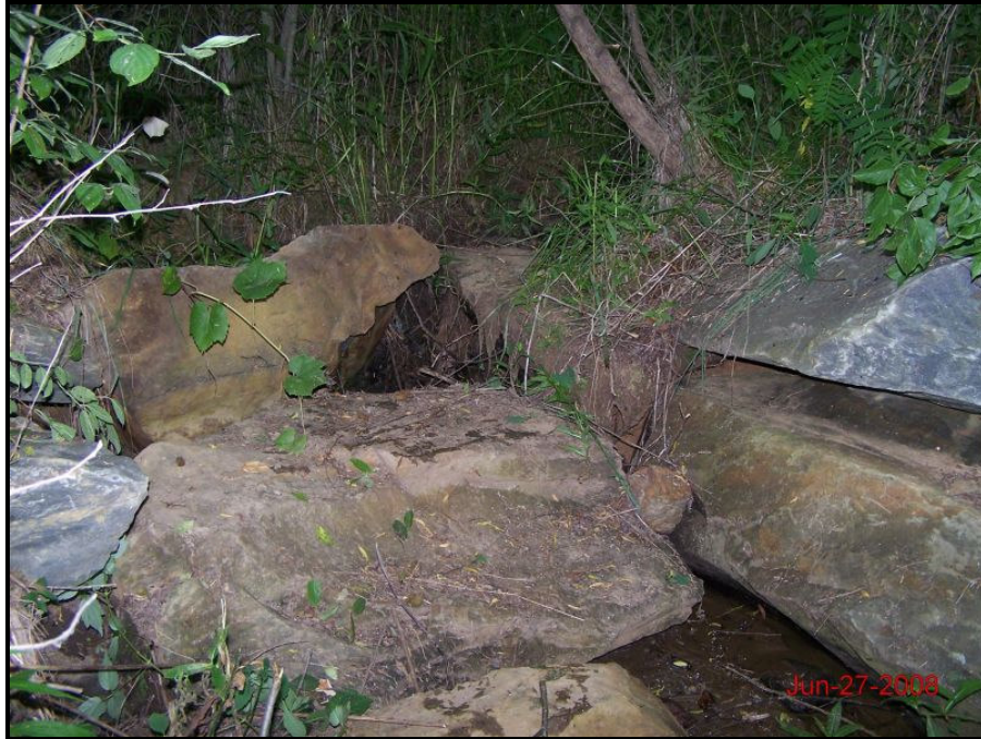
Stream Problem Area (SPA 3) – Failed structure Monitoring Year 4 – June 27, 2008
