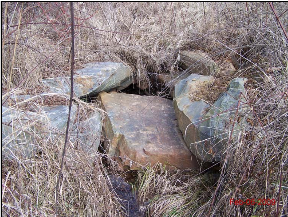
Stream Problem Area (SPA 6) – Failed Structure on Unnamed Tributary Monitoring Year 5 – February 6, 2009
