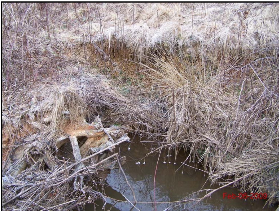
Stream Problem Area (SPA 2) – Bank Erosion Monitoring Year 5 – February 6, 2009
