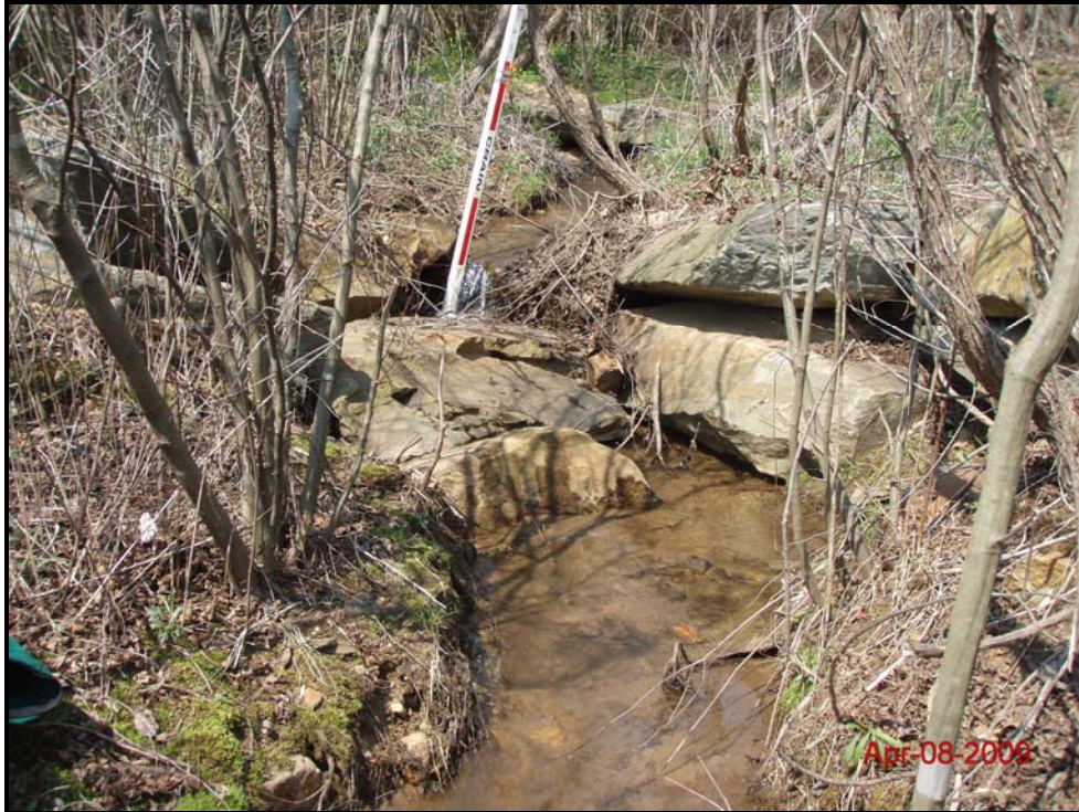
Stream Problem Area (SPA 1) – Pool Aggradation Associated with Stressed Structure Monitoring Year 5 – April 8, 2009
