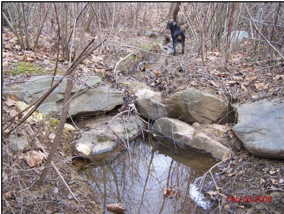
Stream Problem Area (SPA 4) – Stressed Structure Monitoring Year 5 – February 6, 2009
